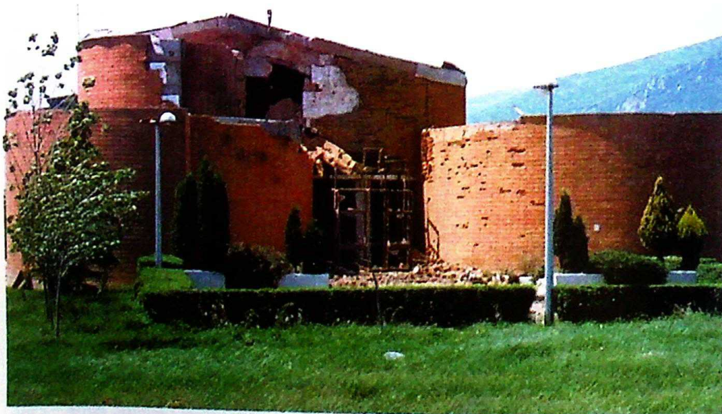
Photo 3 One of the damaged buildings within the KPD "Dubrava" complex
