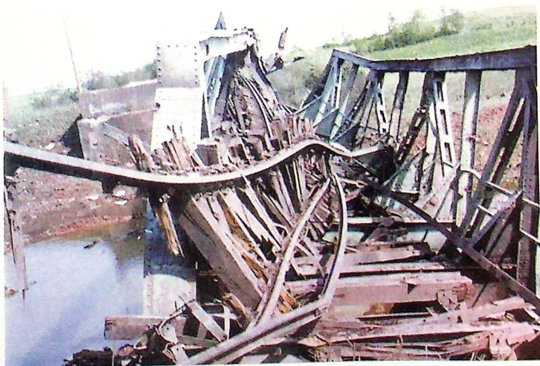
Photo 38 Close-up of the sunken railway bridge in Vatin
