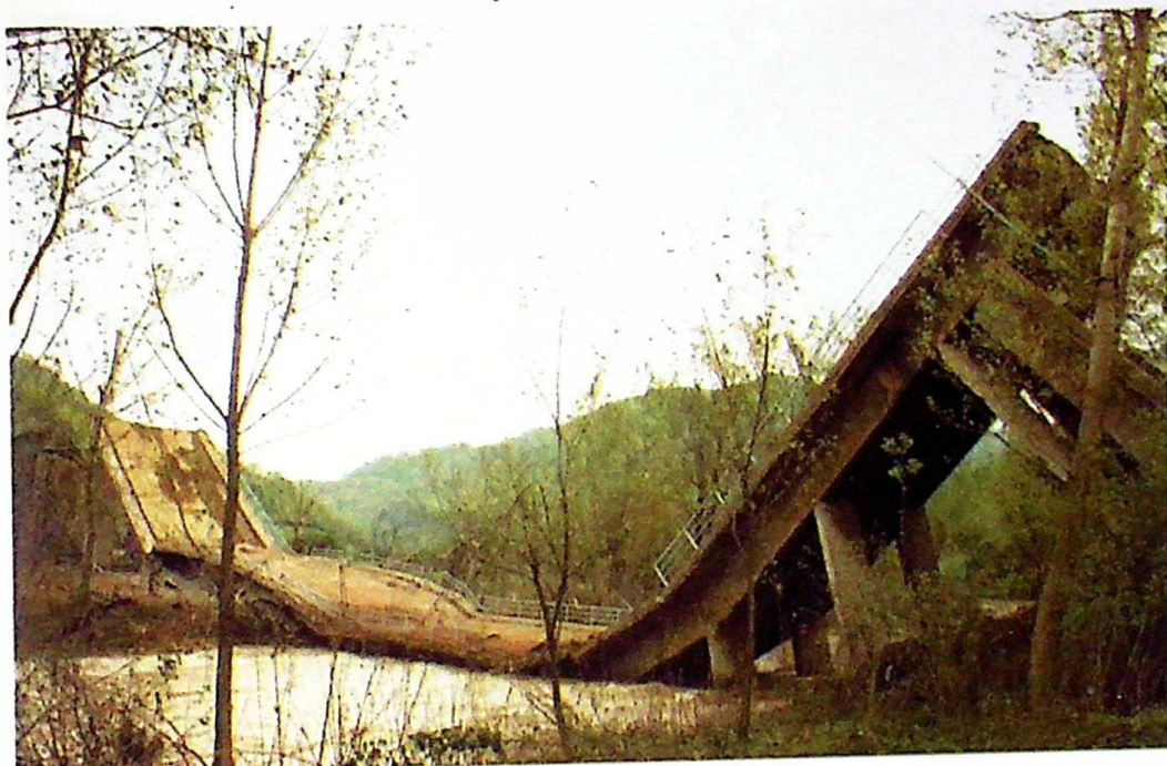
Photo 7 View of the demolished "Sarajevo" bridge in the Grdelica Gorge, on the Leskovac-Vranje road, photographed on 29 April 1999 (Fourth attack)
