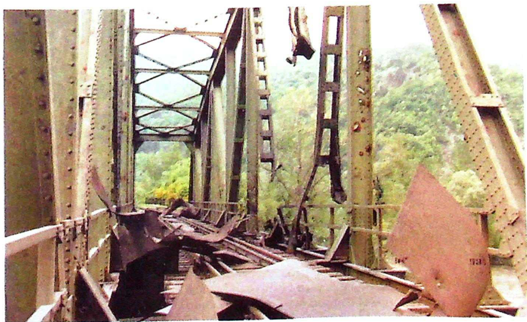
Photo 40 Damaged railway bridge across the Ibar in the village of Bogutovac – Kraljevo, on the Kraljevo–Kosovo Polje railway line, photographed on 8 May 1999
