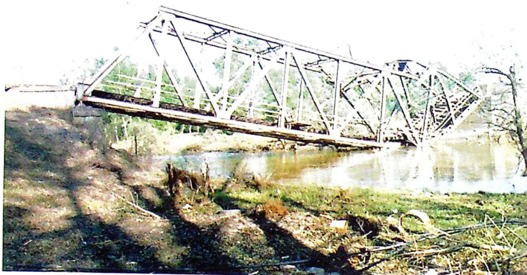
Photo 27 Demolished railway bridge on the Toplica River in the village of Podina – Žitorada – Prokuplje, 2 May 1999
