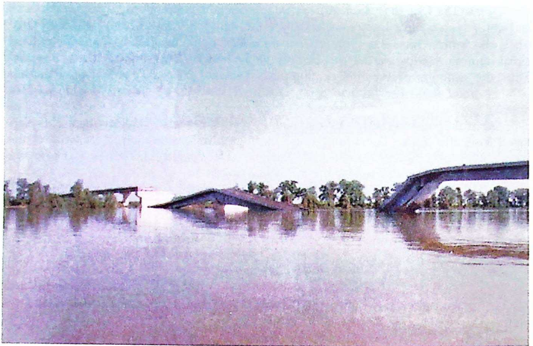
Photo 3 Broad view of the left side of the demolished "Ostružnica" road bridge across the Sava River, 29 April 1999
