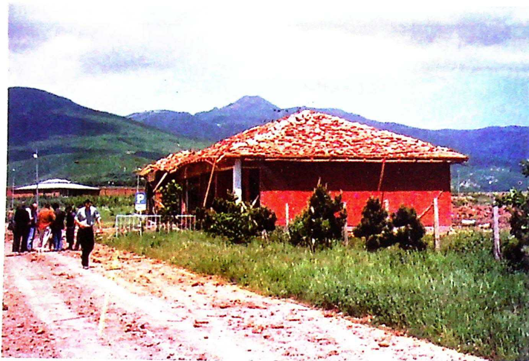
Photo 2 Entrance to the KPD "Dubrava". The destroyed registration office
