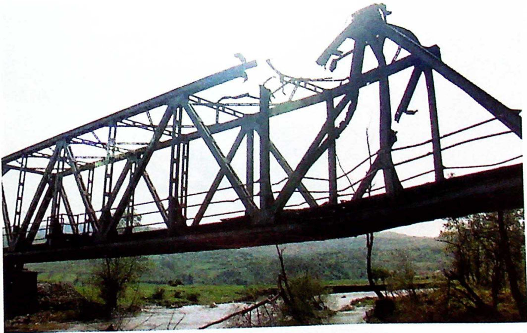
Photo 11 Damaged railway bridge on the river Toplica in the village of Podina, Žitorada – Prokuplje, 29 April 1999 (First attack)
