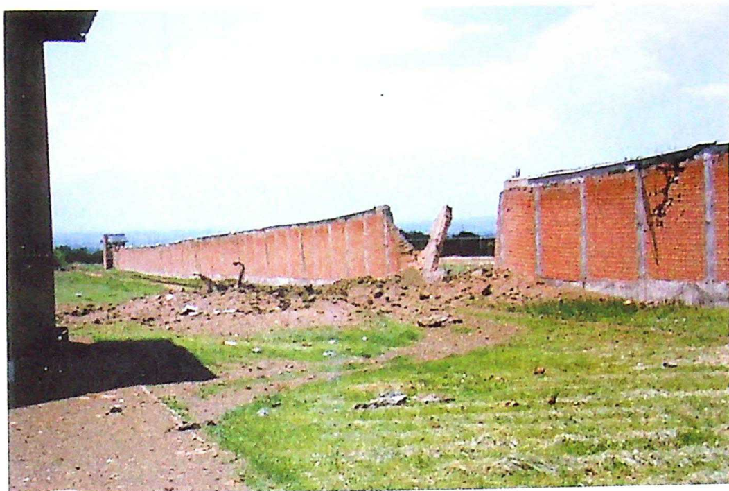
Photo 4 Destroyed section of the KPD "Dubrava" surrounding wall
