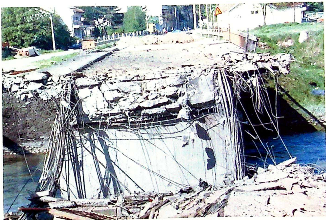
Photo 26 Close-up of the destroyed bridge in the village of Dedina
