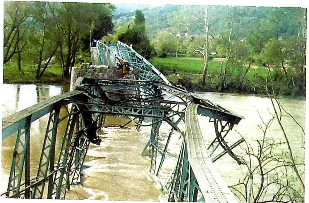
Photo 12 View of the demolished old bridge on the Zapadna Morava River in Trstenik, 30 April 1999
