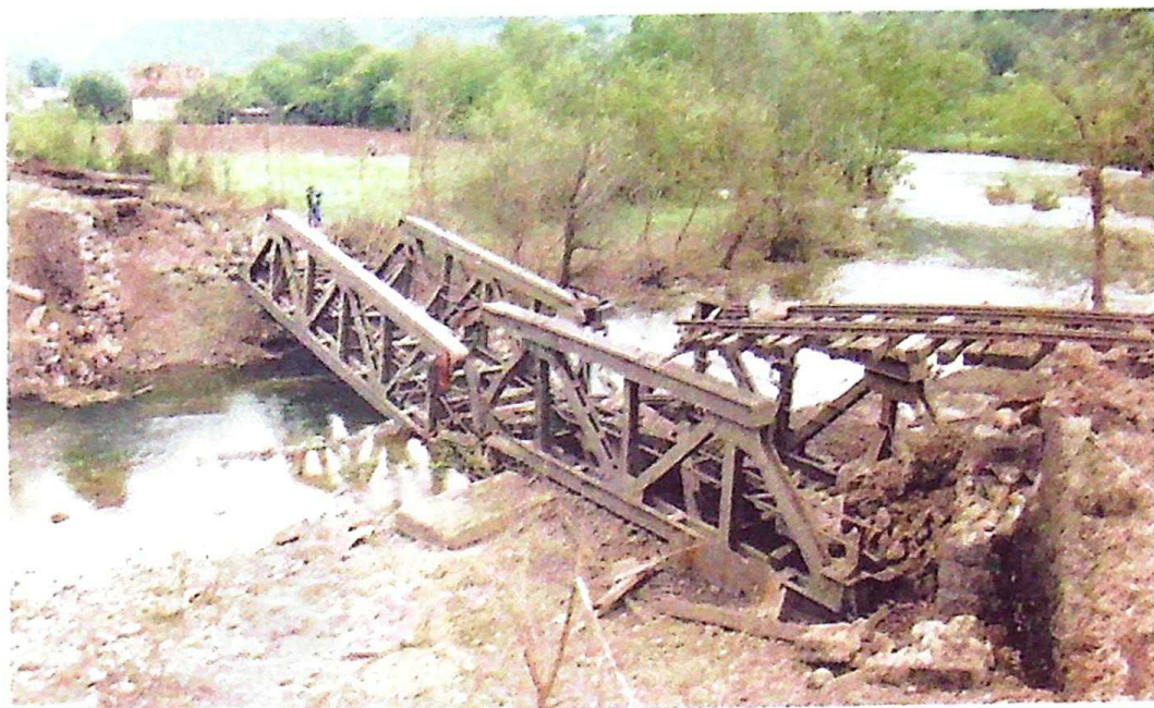
Photo 39 Destroyed railway bridge across the Lopatnica River in the village of Bogutovac – Kraljevo, on the Kraljevo–Kosovo Polje railway line, photographed on 8 May 1999
