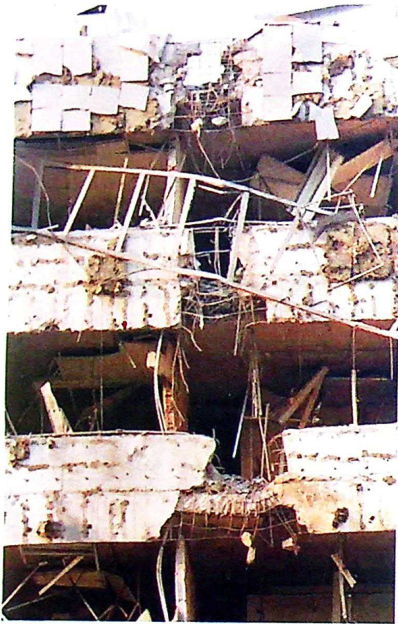
Photo 58 The point of missile impact on the southern facade of the Embassy
