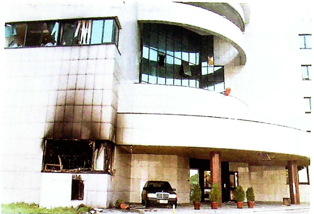
Photo 66 The main entrance to the Embassy with damage from burning
