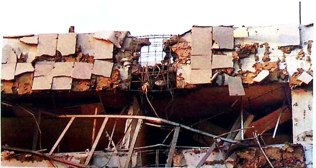
Photo 59 Close-up of the point where the missile struck on the southern facade of the Embassy building
