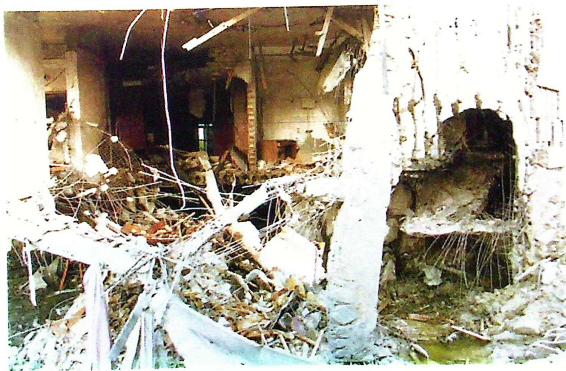
Photo 65 The point of impact between the main and the auxiliary buildings
