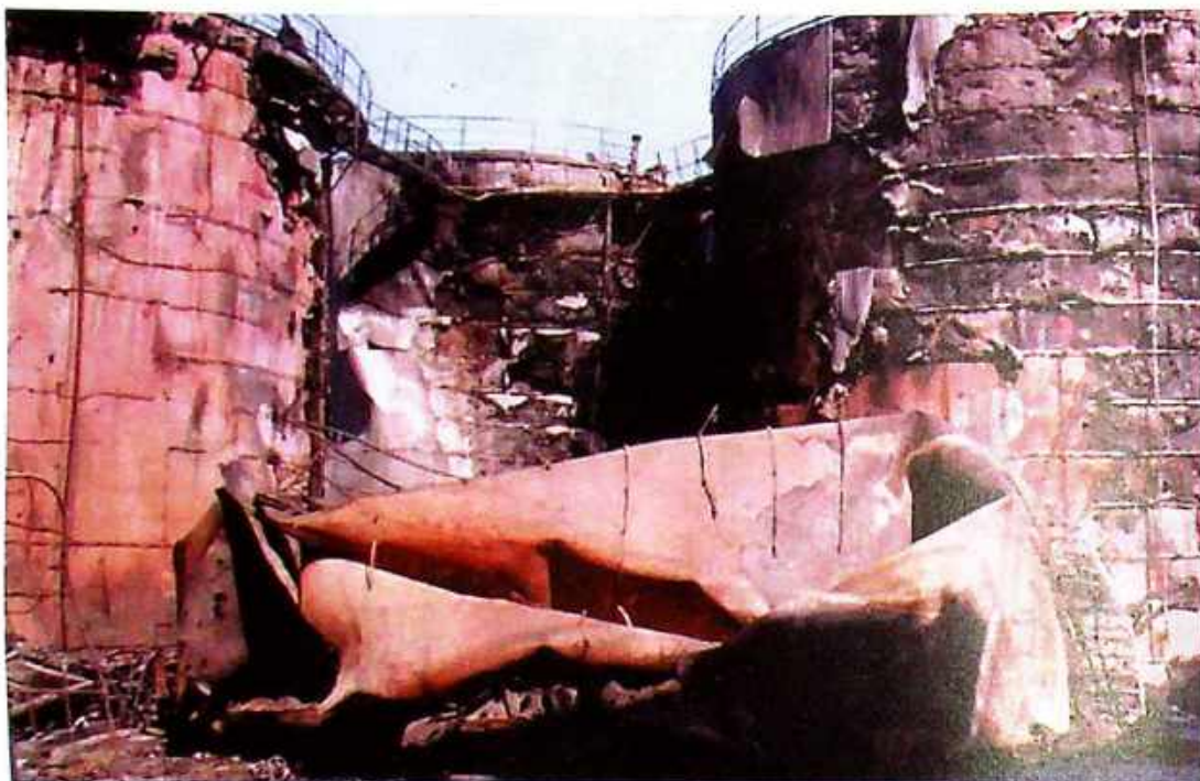
Photo 12 Close-up of damaged oil storage tanks of NIS, Novi Sad
