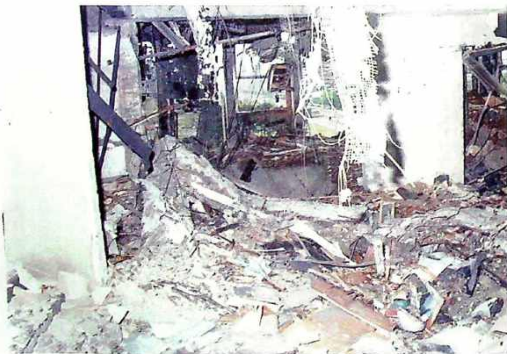
Photo 32 The site where the missile entered the premises of RTV "Košava" in the "Ušće" business center building
