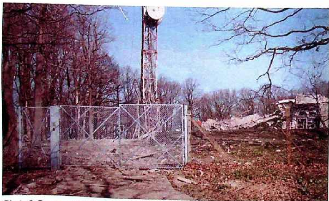
Photo 3 Damaged "Crveni Čot" transmitter on Mt. Fruška Gora.
