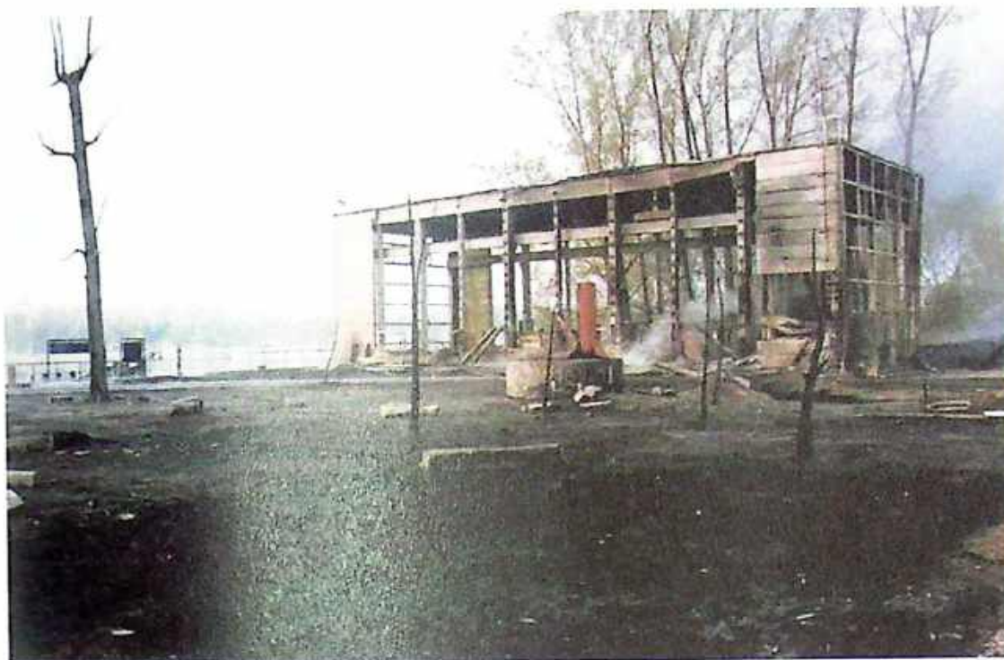
Photo 14 Damaged pumping unit – "Beogradske elektrane", Novi Beograd
