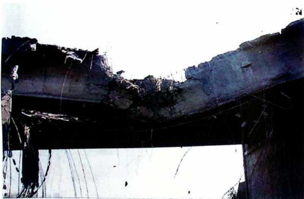
Photo 16 Close-up of the point of damage
