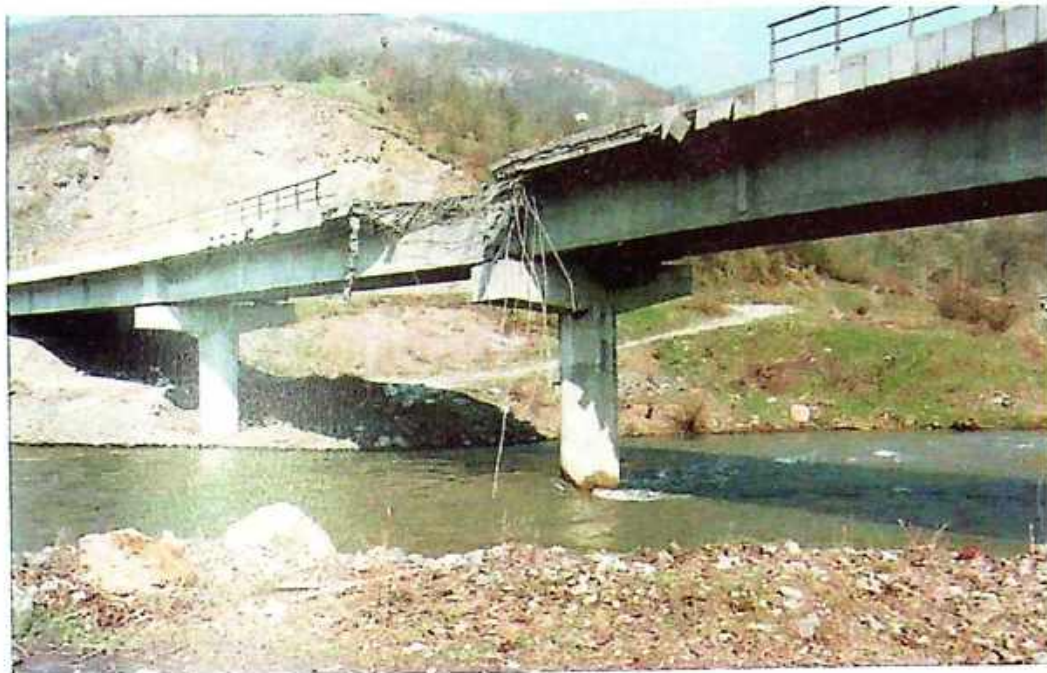
Photo 13 Damage of the bridge across the Ibar river in the village of Biljanovac, Kraljevo Municipality
