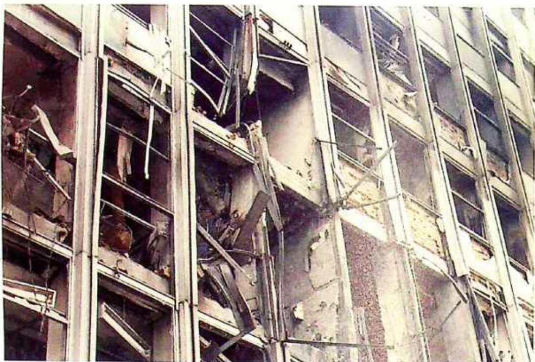
Photo 27 Outside view of the damaged second and third floors of "Ušće" business center where the missile entered
