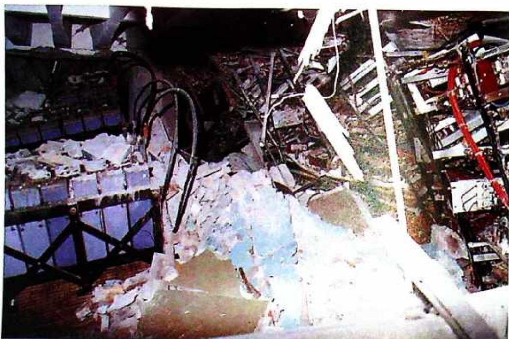
Photo 69 Damaged battery station in the post office
