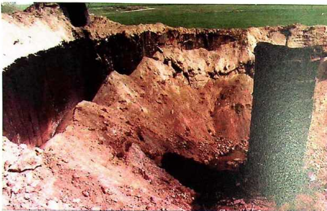
Photo 9 View of the destroyed shaft and supporting pillar of oil storage tank No. 3
