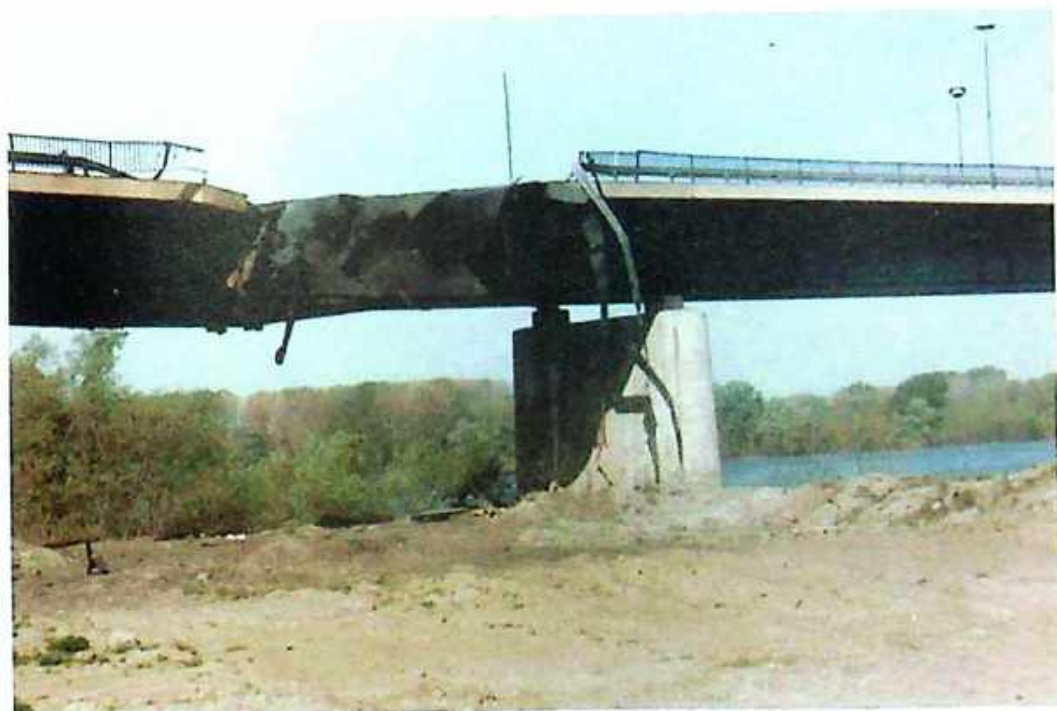
Photo 64 Broad view of the damaged bridge from the Smederevo side
