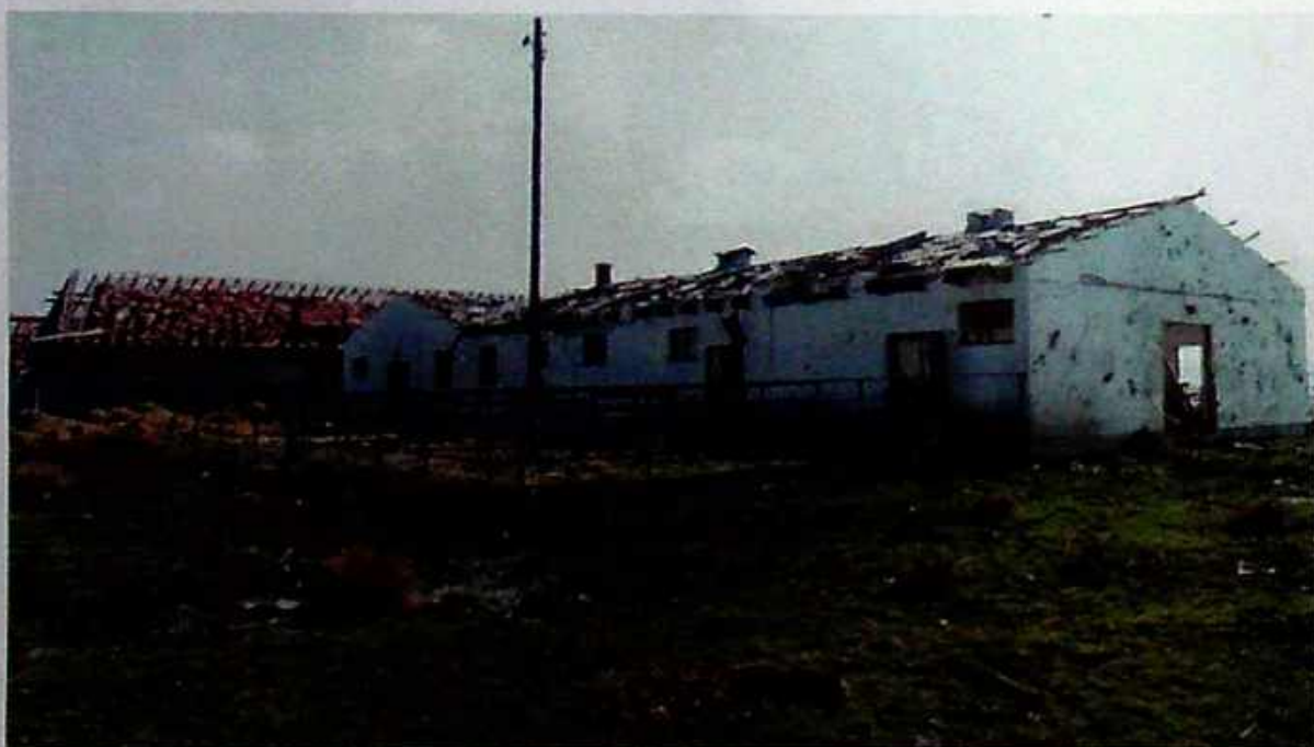
Photo 35 Demolished facilities belonging to Agricultural-Industrial Complex PIK "Pešter" in the village of Dubinje, municipality of Sjenica
