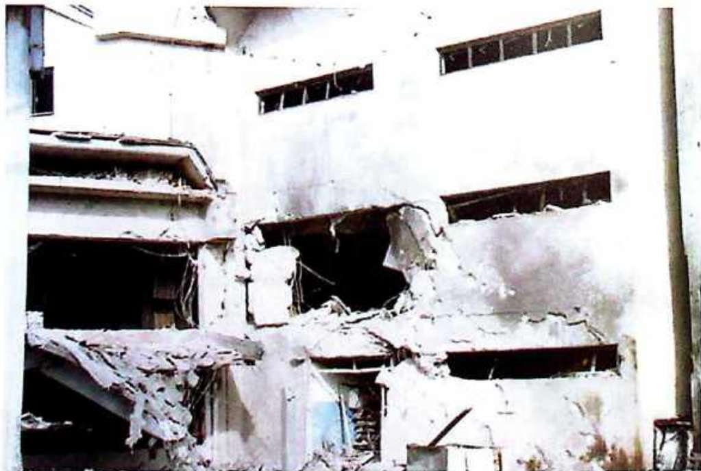
Photo 34 Close-up of the point where a missile struck the bus station
