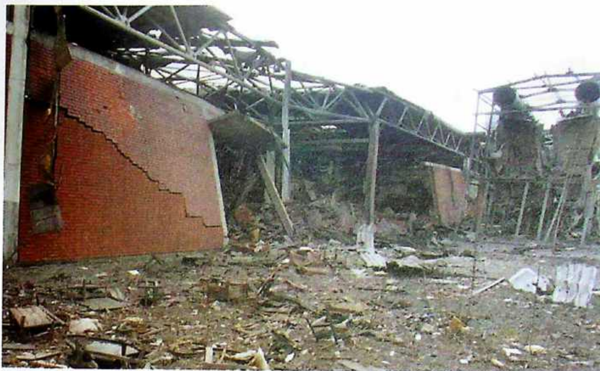
Photo 42 Destroyed accumulator production plant - "Krušik", Holding Corporation, Valjevo, 14 April 1999
