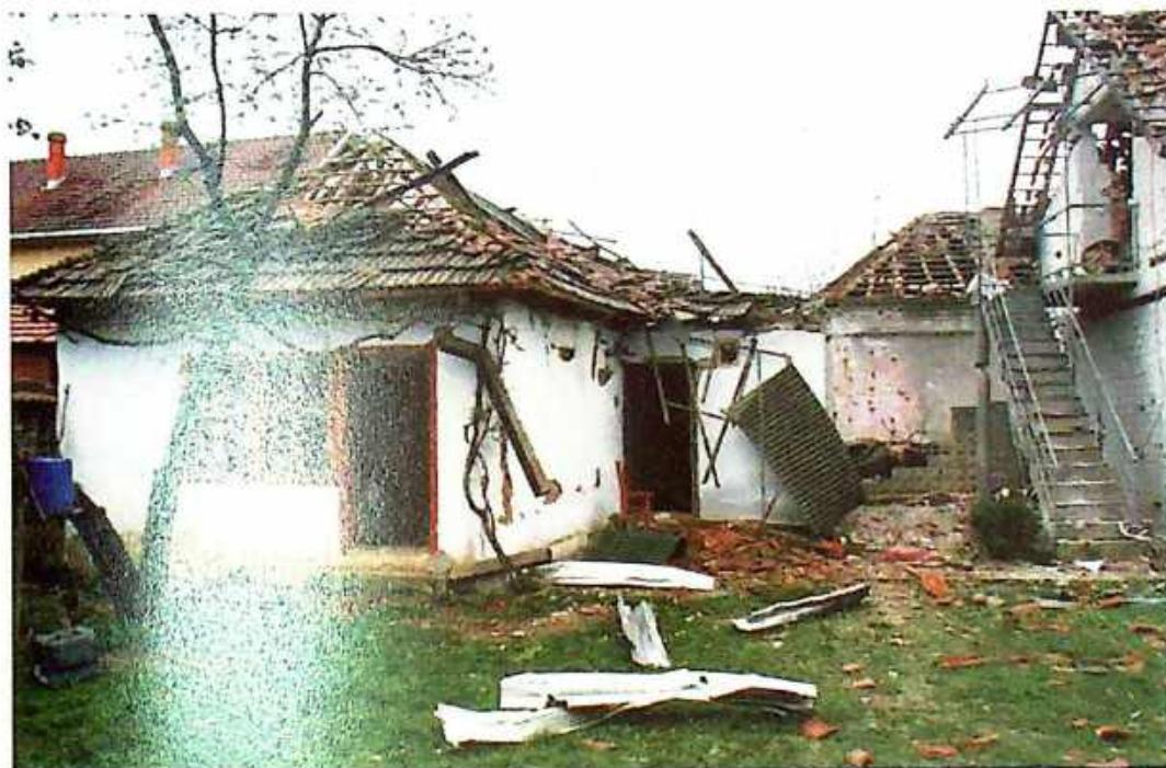
Photo 47 Damaged houses in Turekovac village, Leskovac municipality
