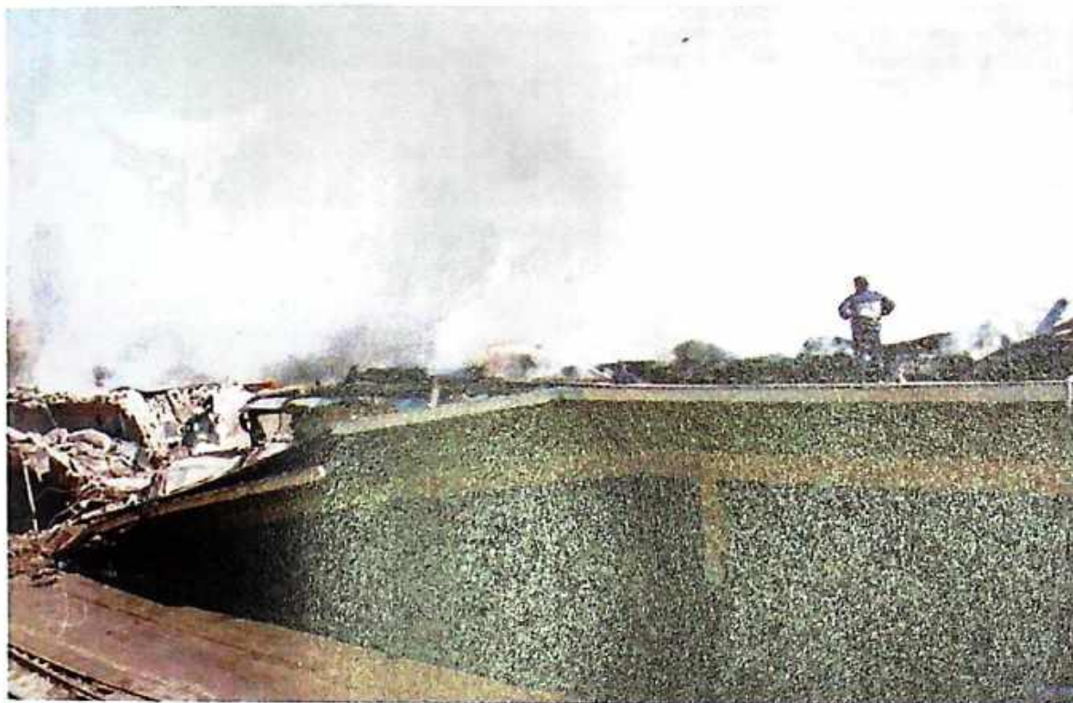
Photo 18 View of the demolished storehouse of tobacco in Niš
