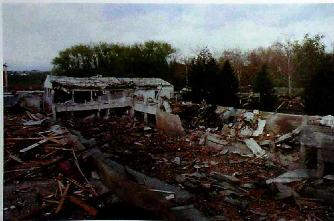
Photo 41 Destroyed cafeteria of "Krušik" Holding Corporation
