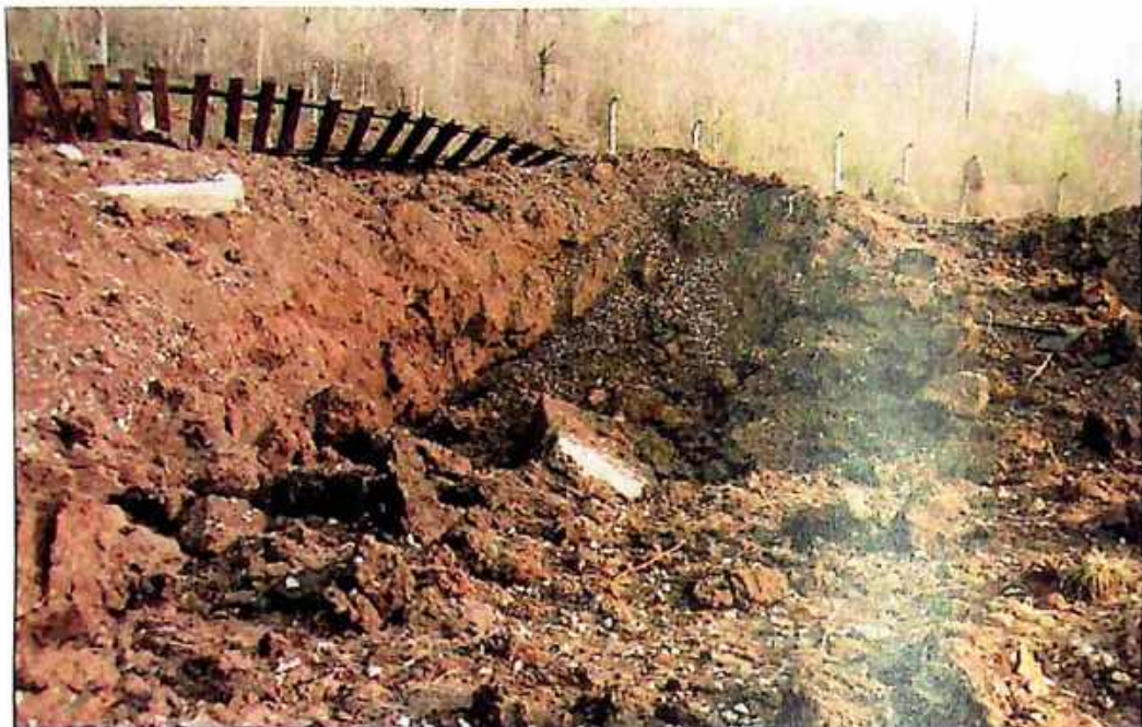
Photo 26 Damaged Kraljevo-Lapovo railway with a crater in the village of Vitanovac, Kraljevo Municipality
