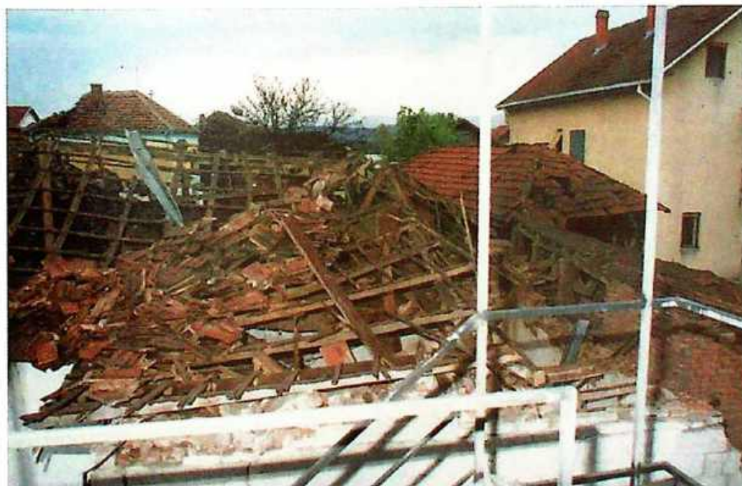
Photo 48 Damaged house of Zoran Nikolić in Turekovac village
