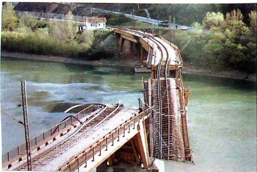
Photo 62 Close-up of the sunken bridge
