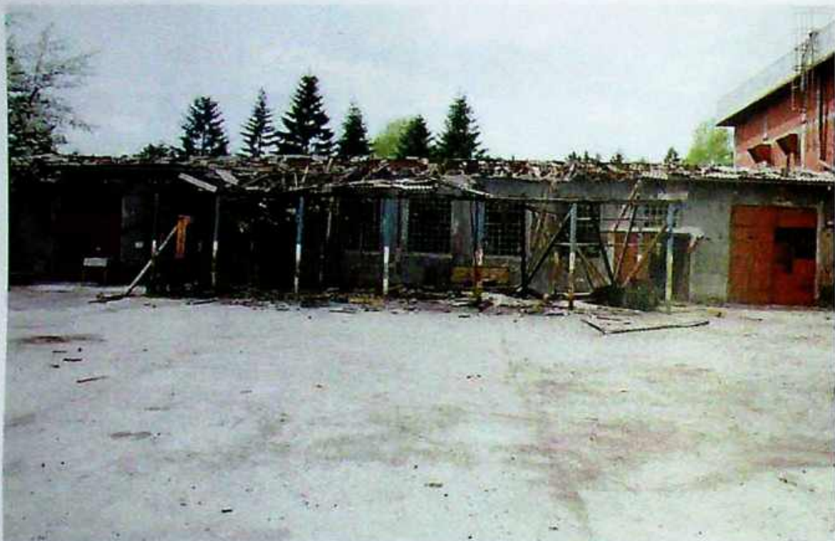
Photo 40 Destroyed vehicle shed
