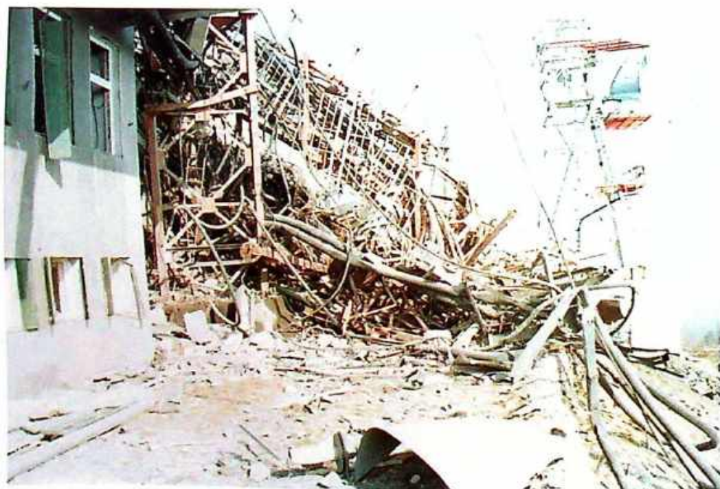
Photo 13 View of destroyed aerial system of the repeater
