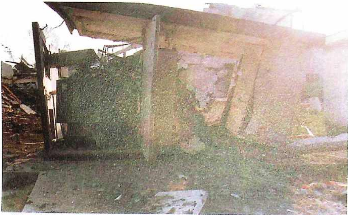
Photo 31 Close-up of damaged "Fuel 2" facility
