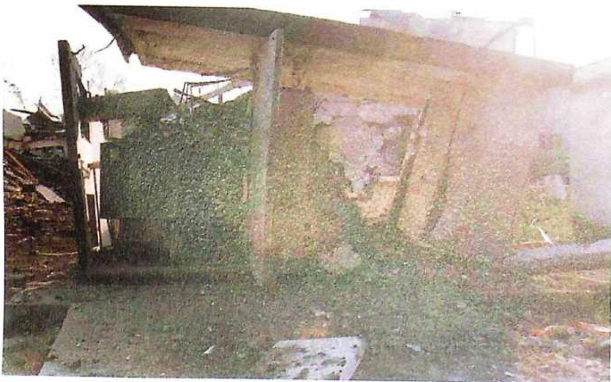
Photo 31 Close-up of damaged "Fuel 2" facility
