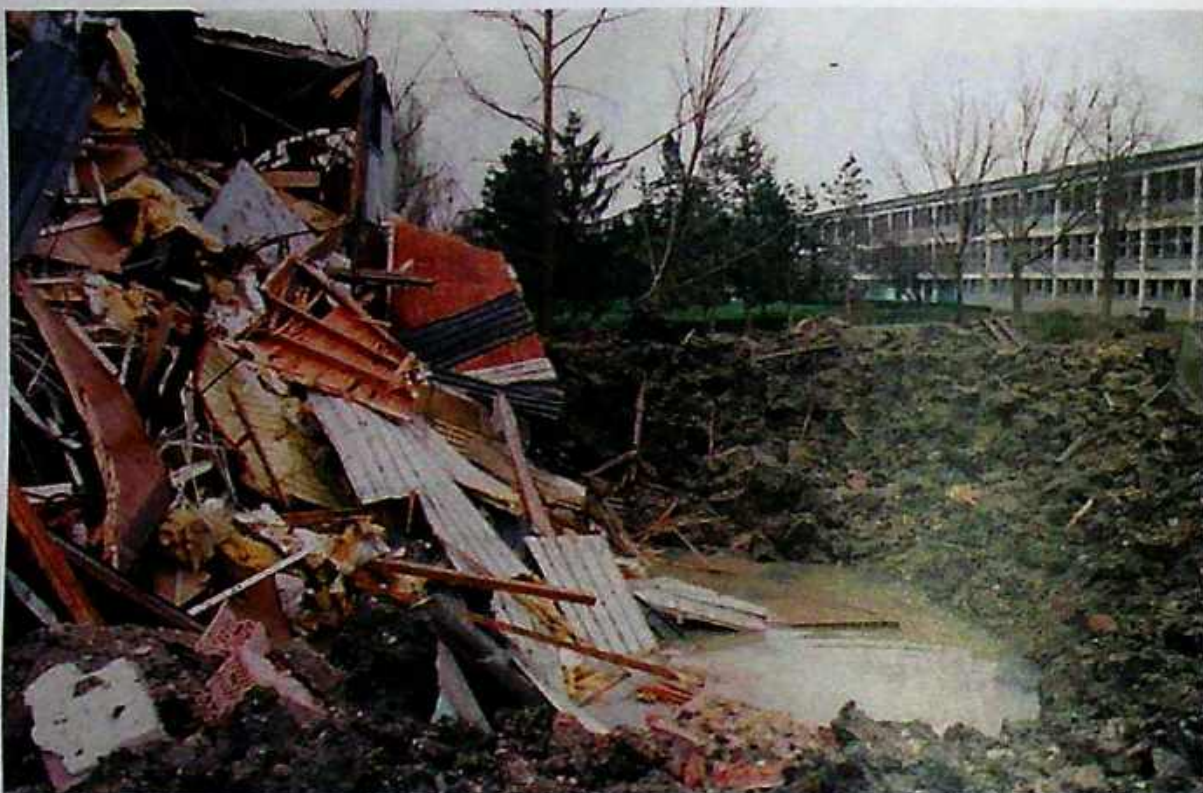
Photo 34 Close-up of the demolished Computer Center building with crater
