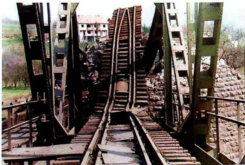
Photo 24 Close-up of the damaged bridge
