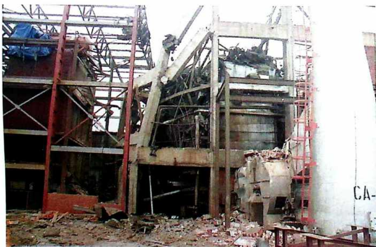
Photo 2 Damaged boiler room and boiler No. 3 in energy plant, NIS oil refinery in Pančevo
