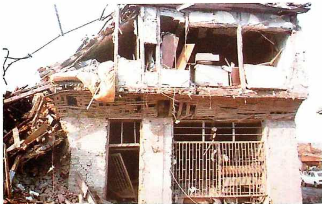
Photo 36 One of the demolished houses in the vicinity of Priština Post Office, April 7, 1999
