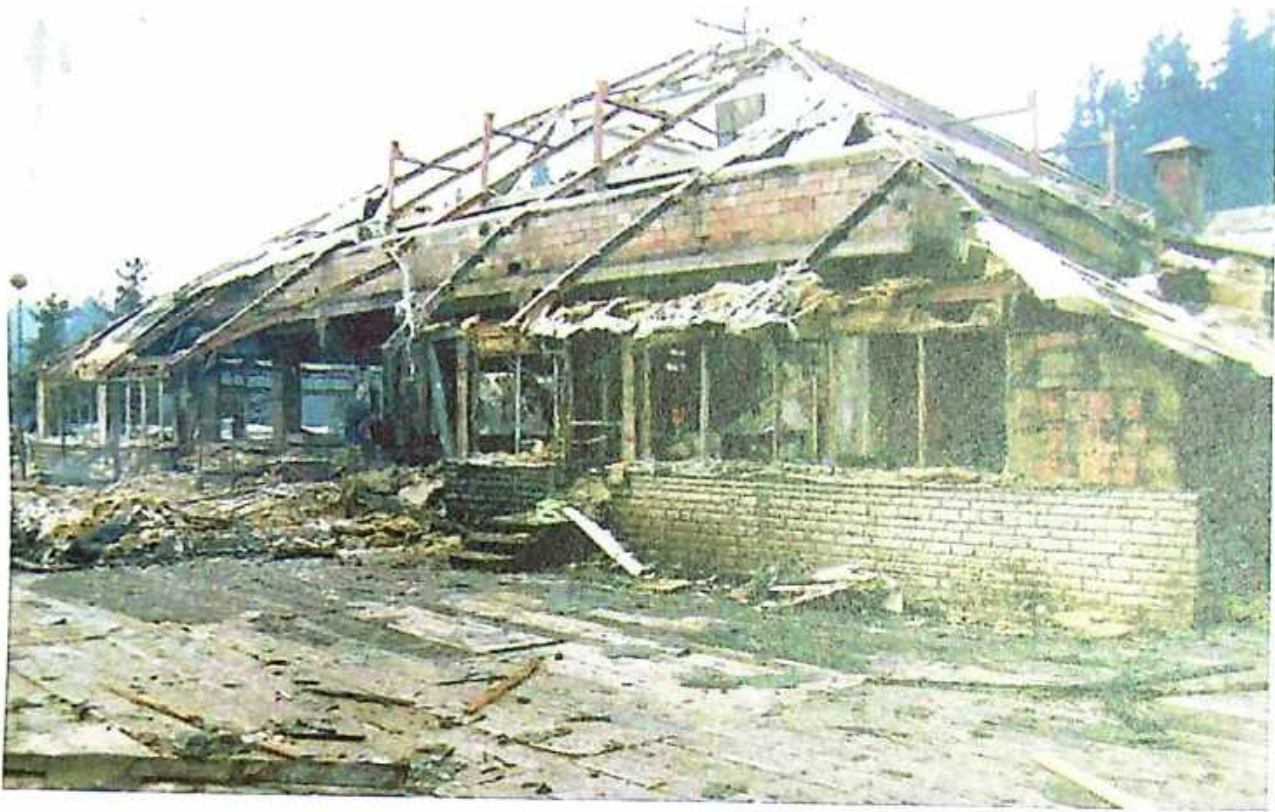
Photo 7 Demolished and burned restaurant of hotel "Bačiste" on Mt. Kopaonik
