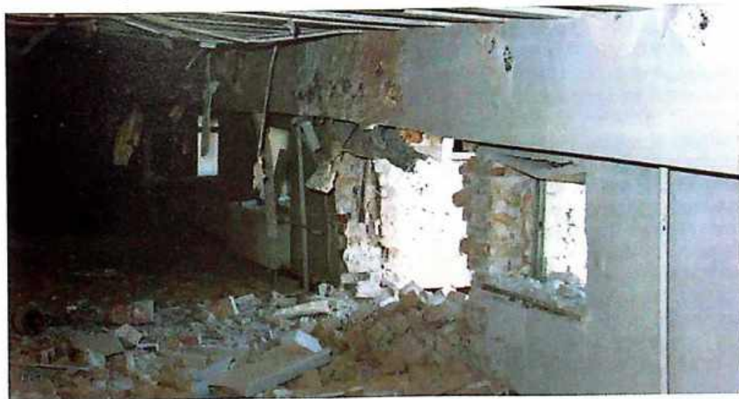
Photo 3 The interior of the Executive Council building at the point struck by a missile
