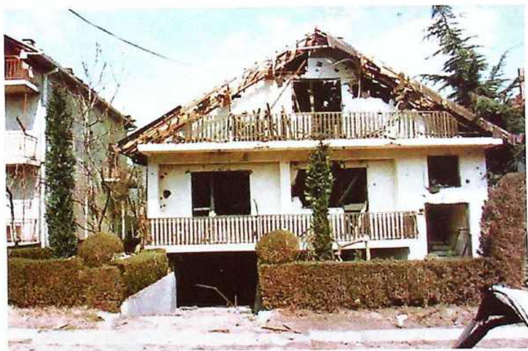
Photo 14 Damaged private house in Vranje
