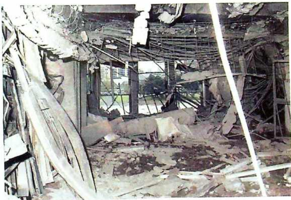
Photo 26 Damaged first floor of "Ušće" business center
