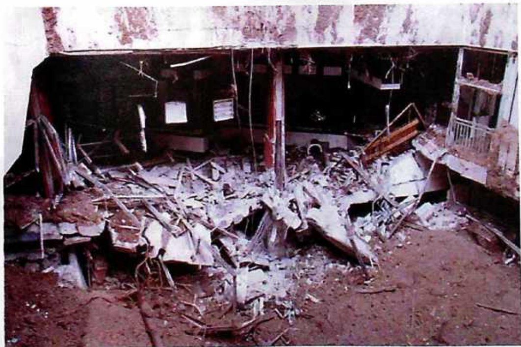
Photo 68 The crater inside the post office building
