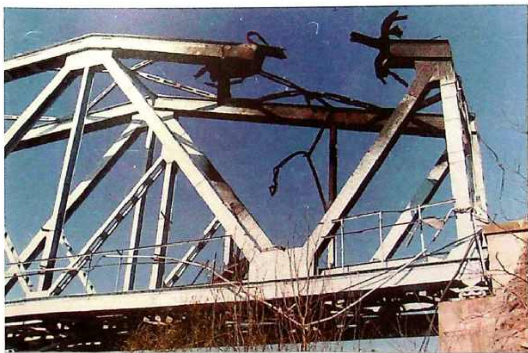
Photo 22 Damaged railway bridge on the Danube in Bogojevo
