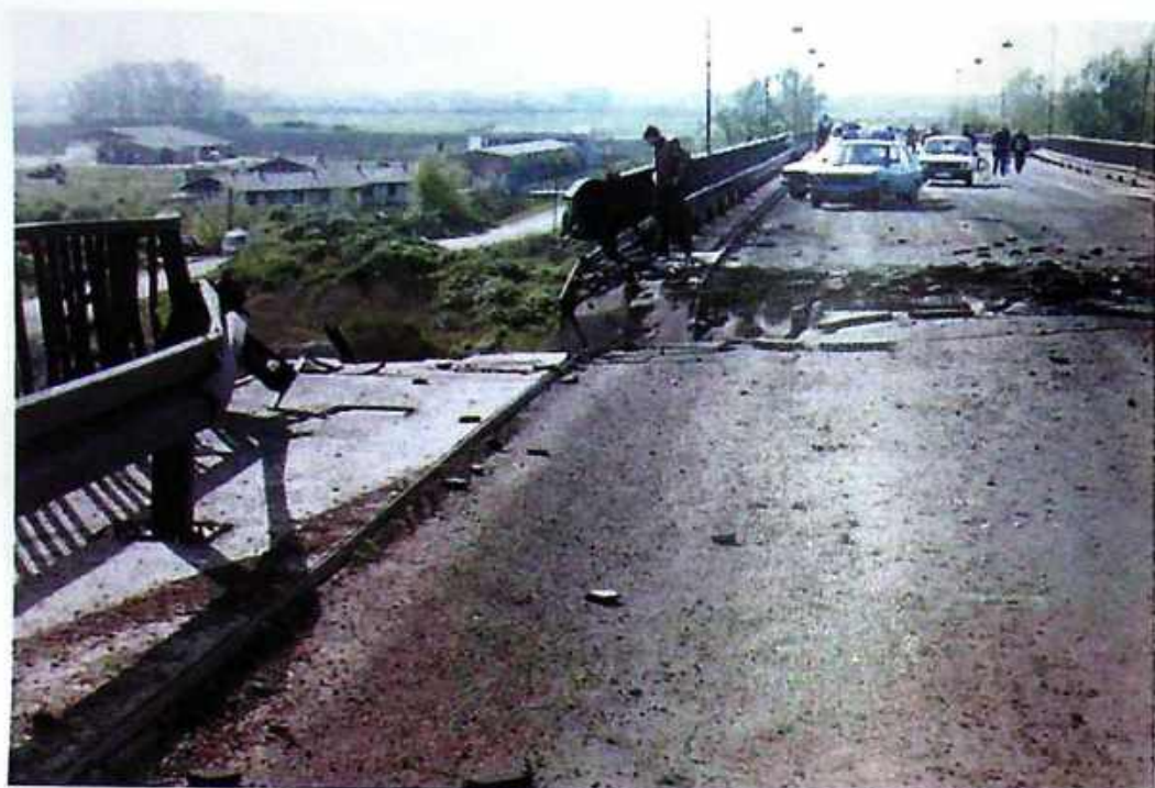
Photo 65 Damaged carriageway of the bridge on the Smederevo side
