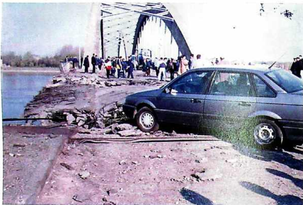
Photo 15 Damaged Petrovaradin railway bridge in Novi Sad
