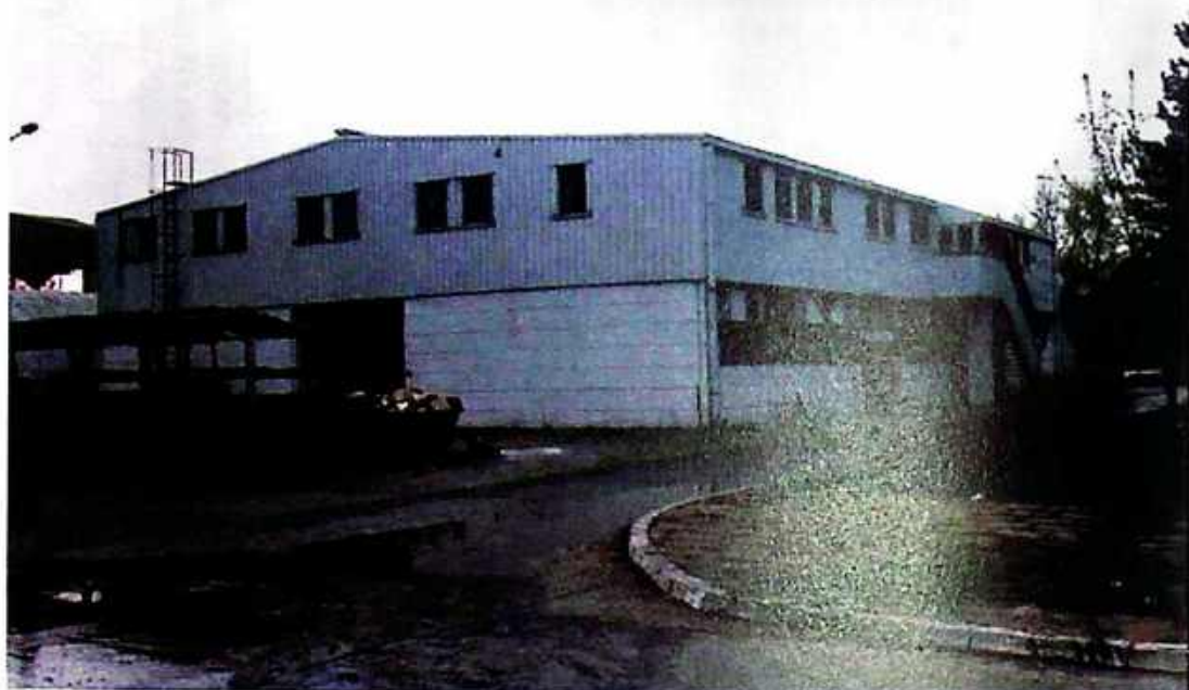
Photo 16 Damaged depots – "Beogradske elektrane", Novi Beograd
