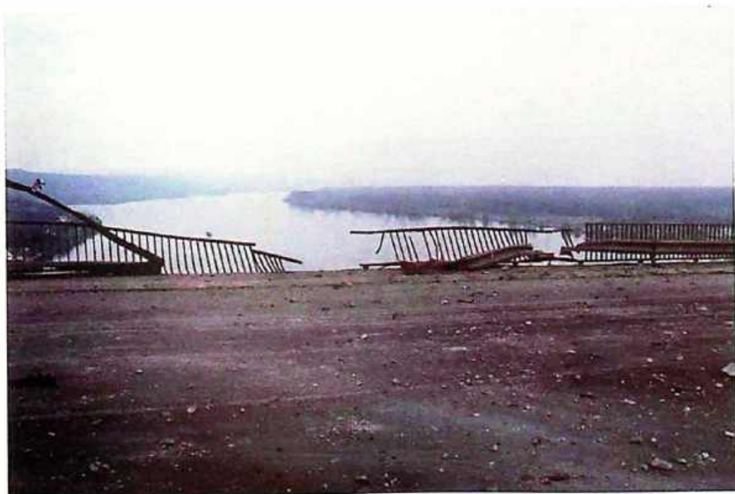
Photo 4 Damaged Beška Bridge opposite the point of impact
