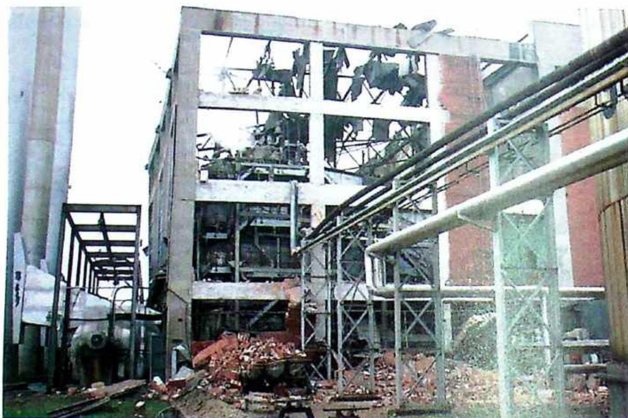
Photo 1 Damaged energy plant, NIS oil refinery in Pančevo
