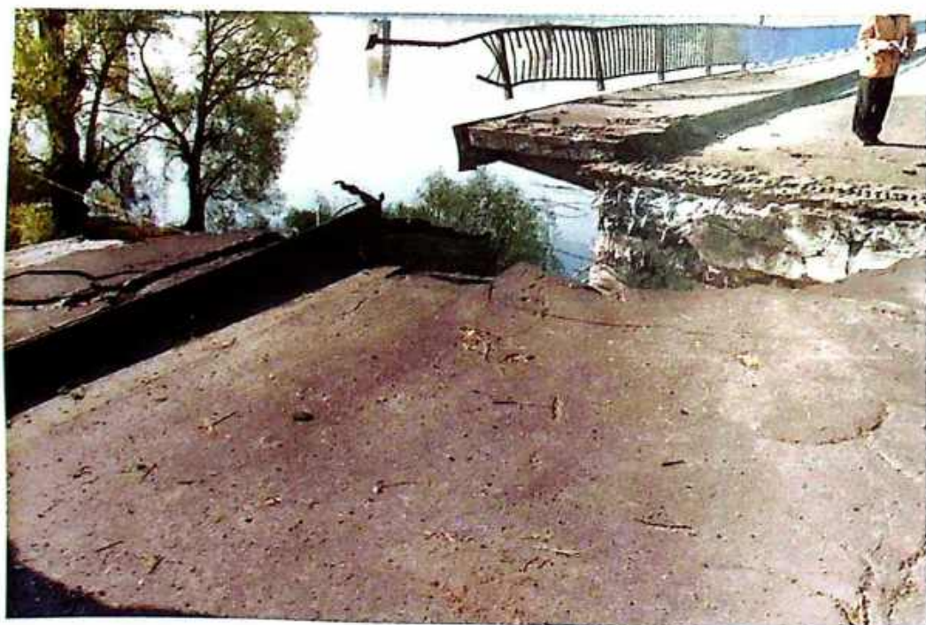
Photo 20 Close-up of the damaged bridge in Bogojevo
