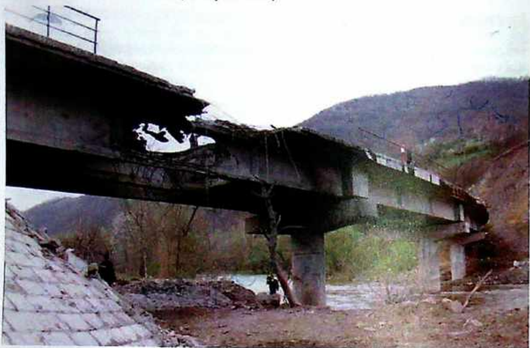
Photo 57 Broad view of the damaged bridge over the river Ibar in the village of Biljanovac, municipality of Kraljevo
