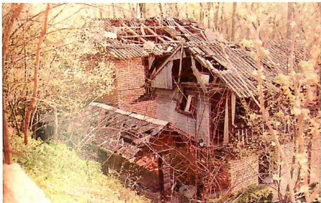
Photo 21 Damaged summer cottage of Branko Vučinić and Vljeko Mladjenović near the Bogojevo bridge
