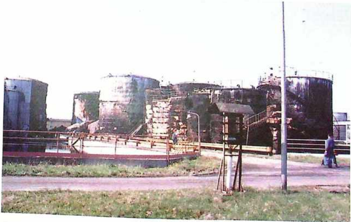
Photo 11 Damaged oil storage tanks within the compound
