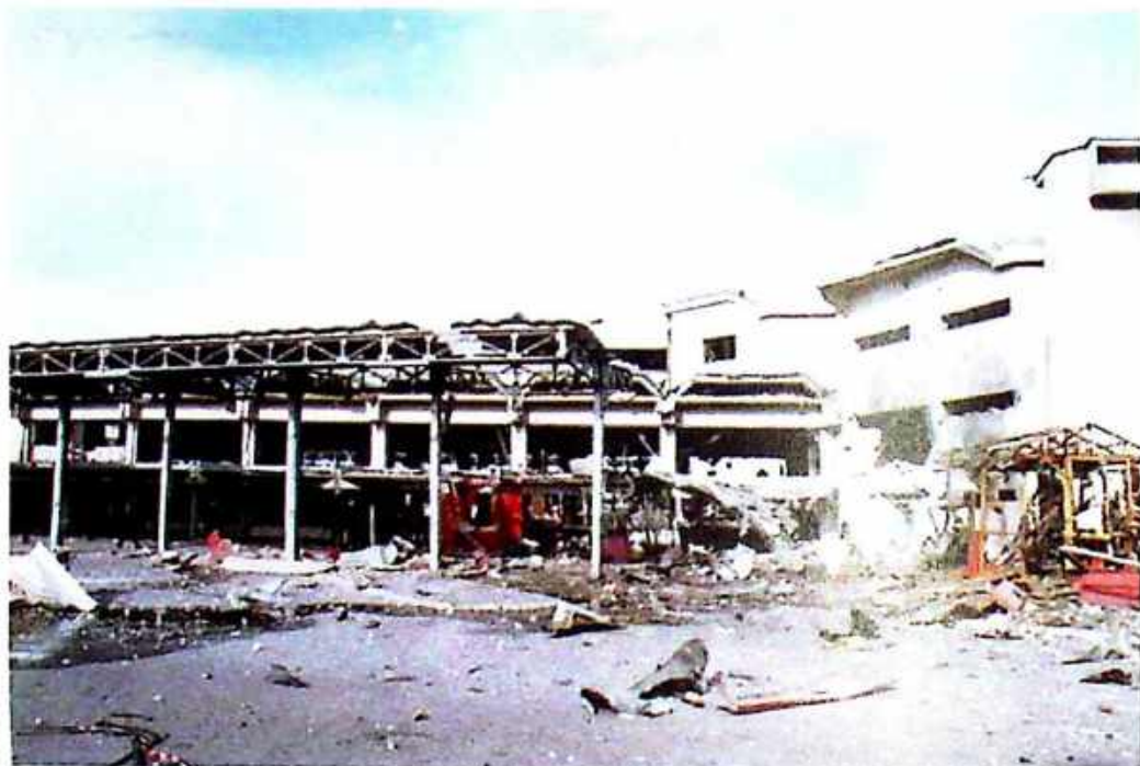
Photo 33 View of the damaged bus station in Priština, 13 April 1999
