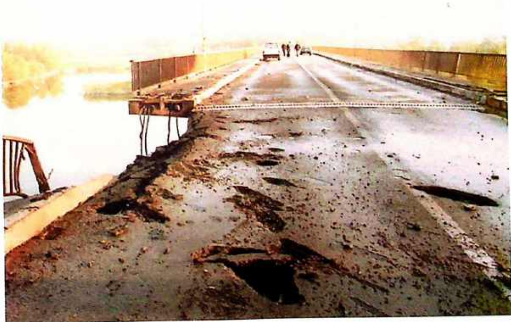
Photo 10 Close-up of the damaged bridge viewed from Bačka Palanka towards Ilok
