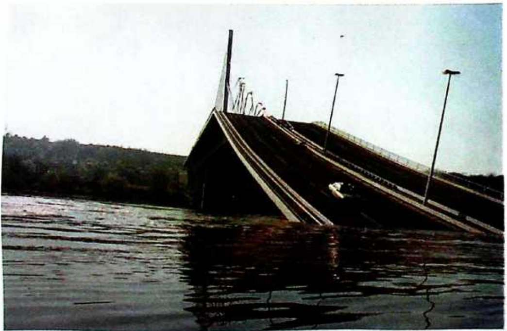
Photo 6 View of the damage from the Srem bank
