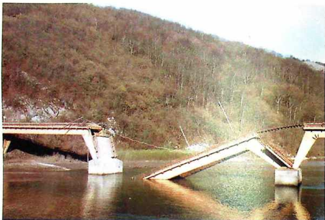
Photo 61 The railway bridge across the Lim in Donja Bistrica sunken on 14 April 1999
