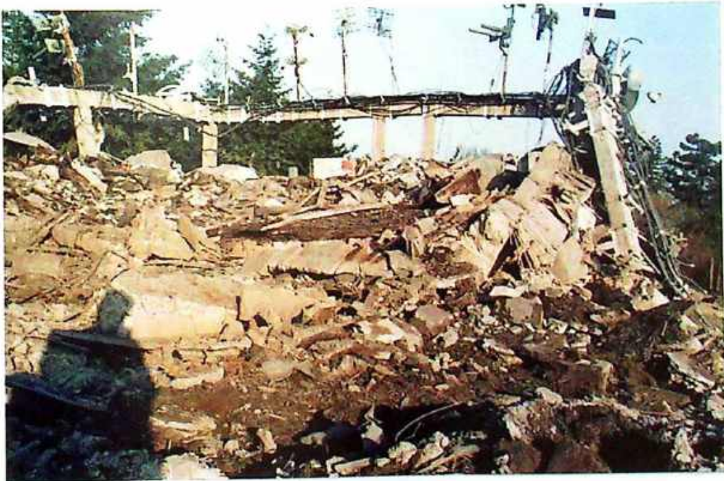
Photo 20 Close-up of the destroyed repeater
