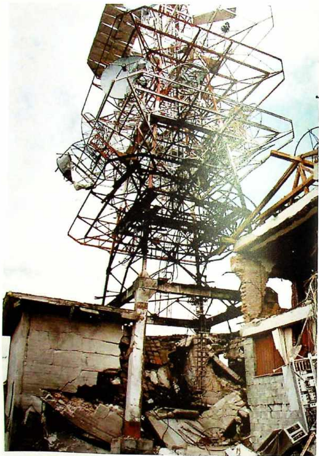
Photo 9 Close-up of the destroyed relay station
