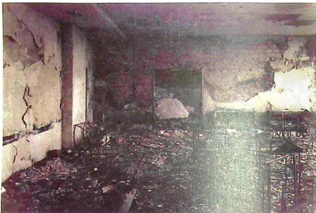
Photo 31 Totally demolished premises of RTV "Košava" on the 23rd floor
