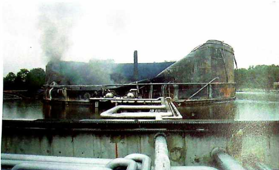
Photo 29 Destroyed crude oil storage tank
