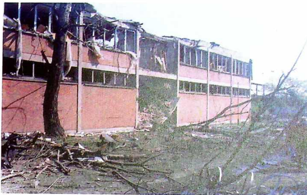
Photo 44 View of damaged administration building of "Prva iskra" Holding in Barič, process equipment factory, municipality of Obrenovac, bombed on 19 April 1999
