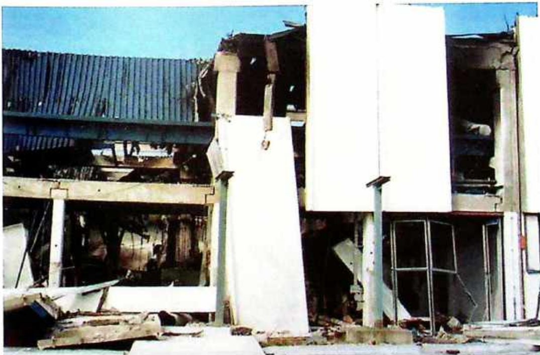
Photo 1 Damaged plant of Lola Utva in Pančevo
