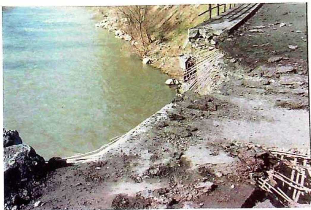
Photo 14 Close-up of the damage on the bridge in Biljanovac
