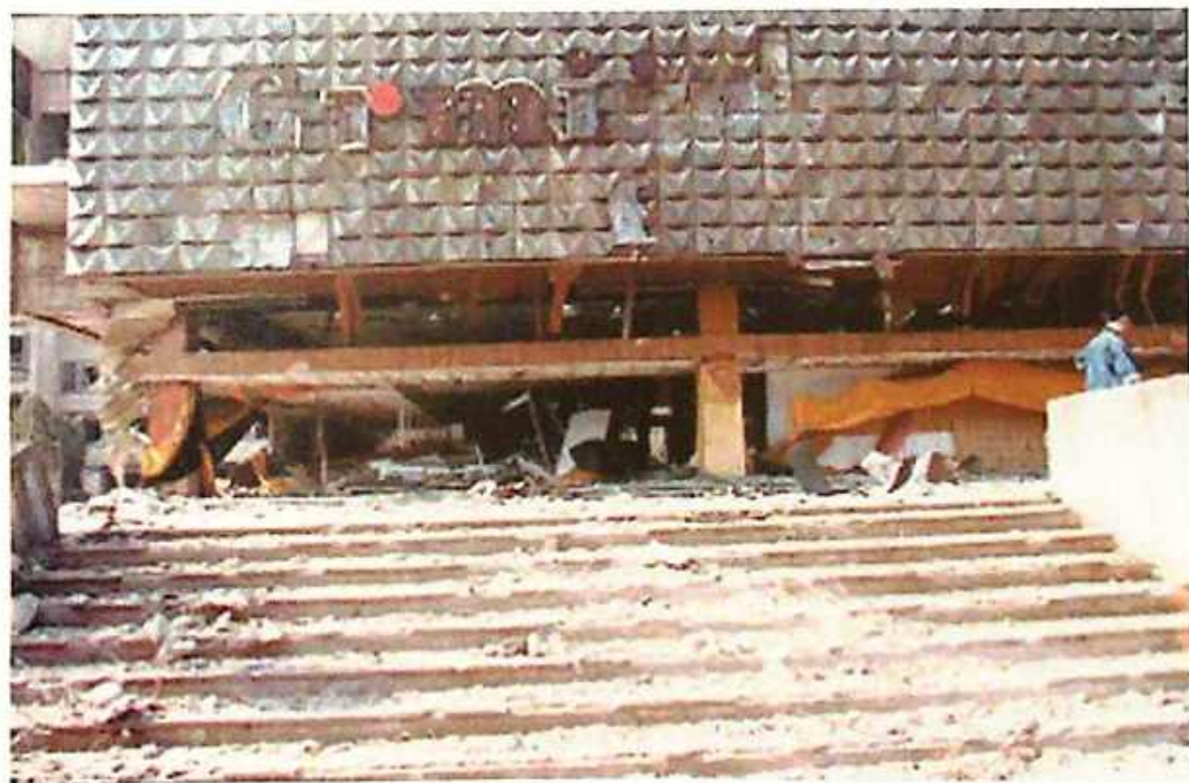
Photo 32 Damaged department store "Grmija" in Priština, April 7, 1999
