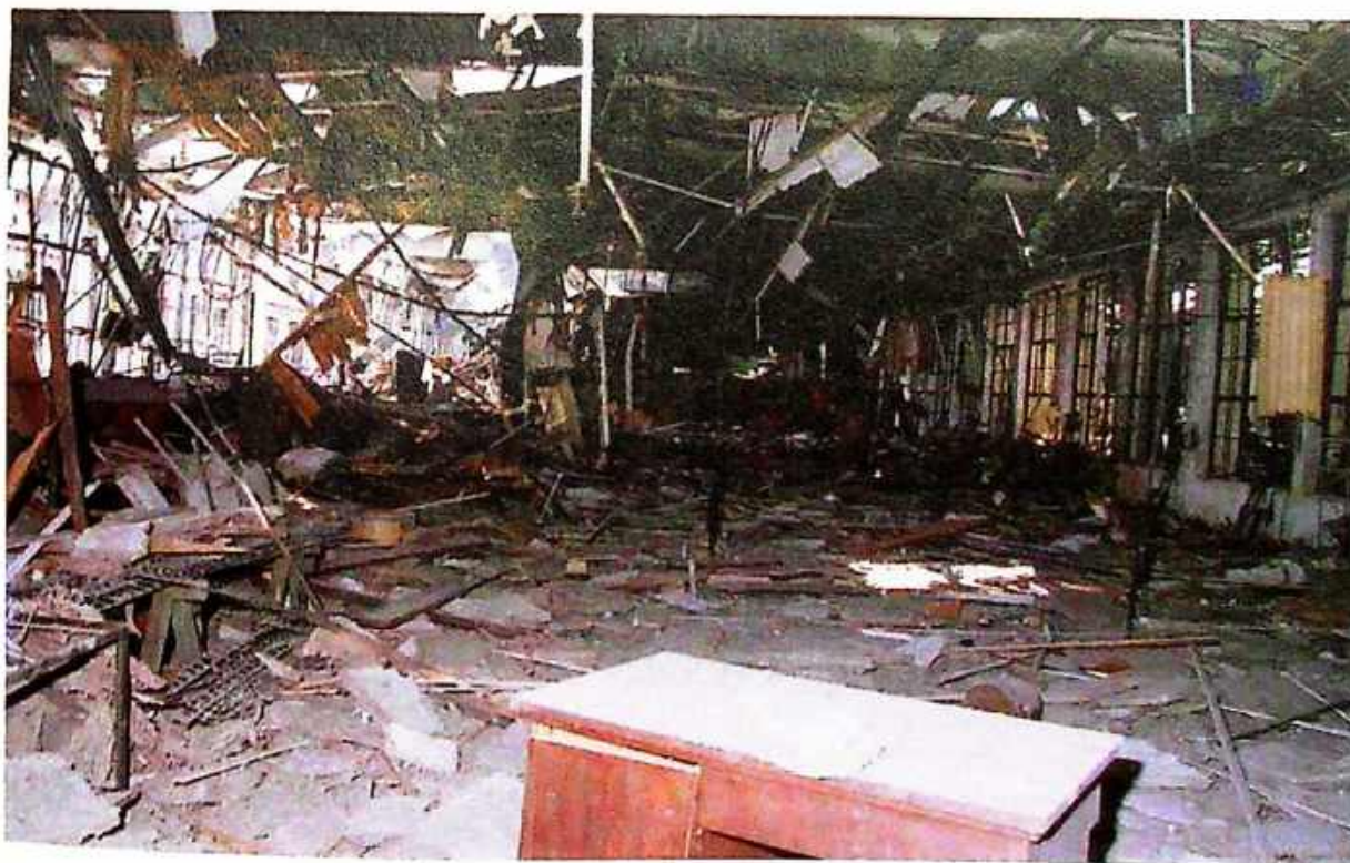
Photo 39 Destroyed textile machines plant in "Krušik" Holding Corporation
