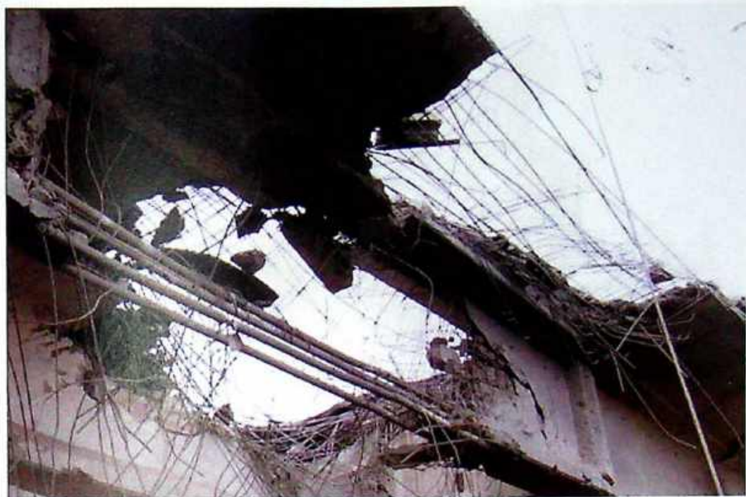
Photo 59 Close-up of the area where the bridge was hit
