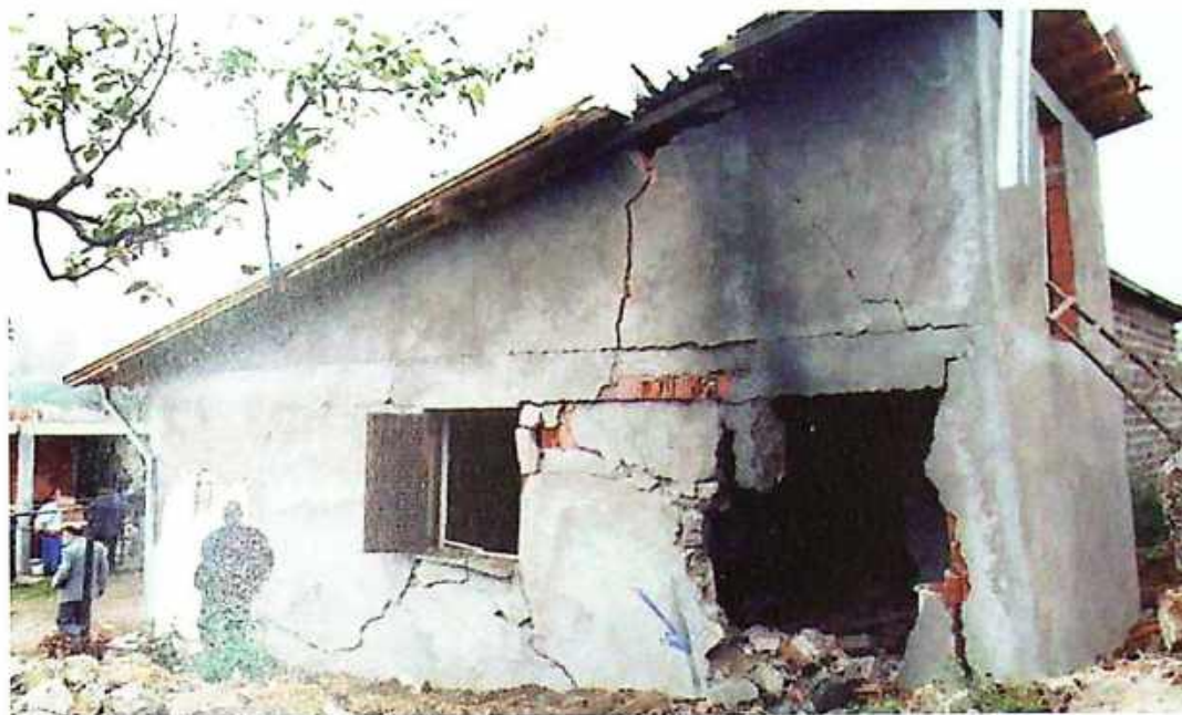
Photo 67 House at 12B Hajduk Veljko St. on Straževica hill, Rakovica municipality, owned by Dragutin Bekčević, damaged by a NATO missile which made a crater next to the house foundation
