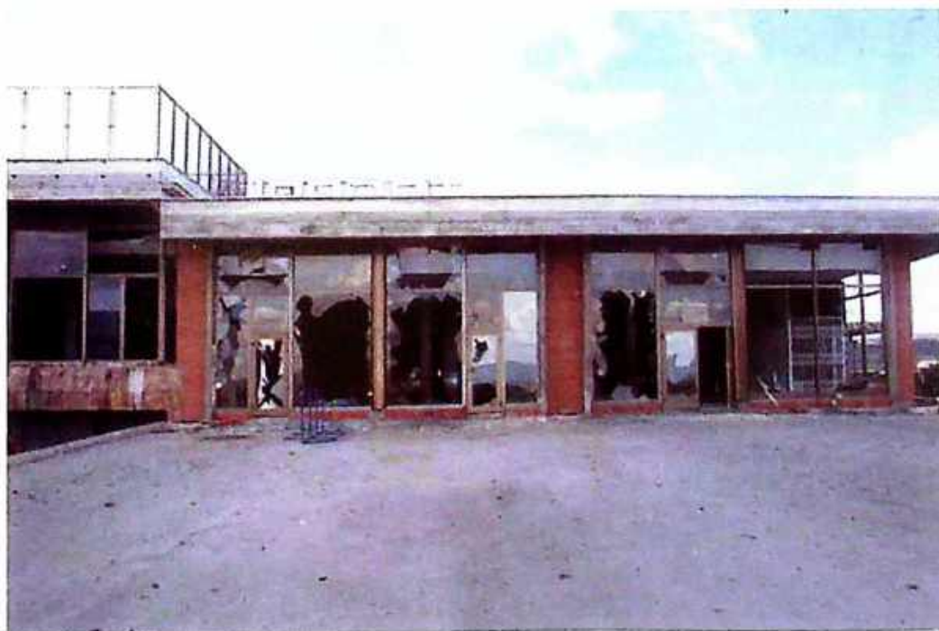
Photo 32 Airport building in Priština damaged on 11/12 April 1999
