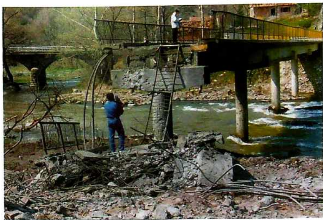
Photo 18 Close-up of the damaged bridge
