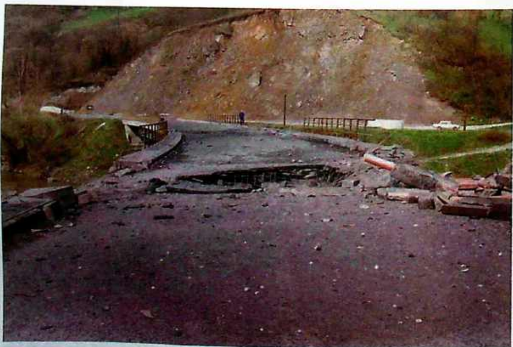
Photo 58 View of the carriageway on the damaged bridge
