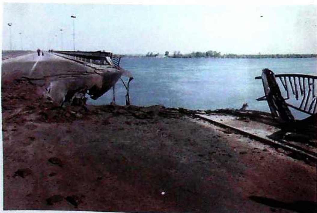
Photo 66 Close-up of the damaged bridge on the Smederevo side
