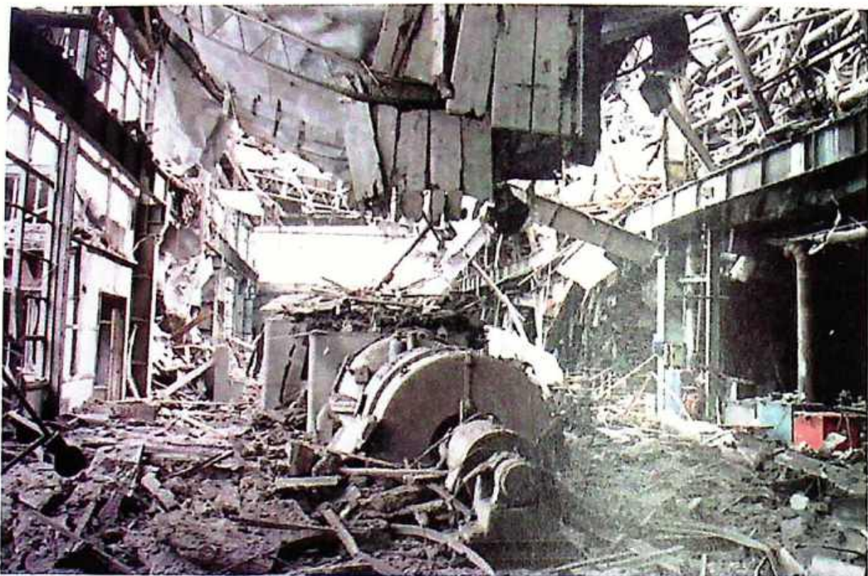
Photo 26 Site where a missile entered the power plant
