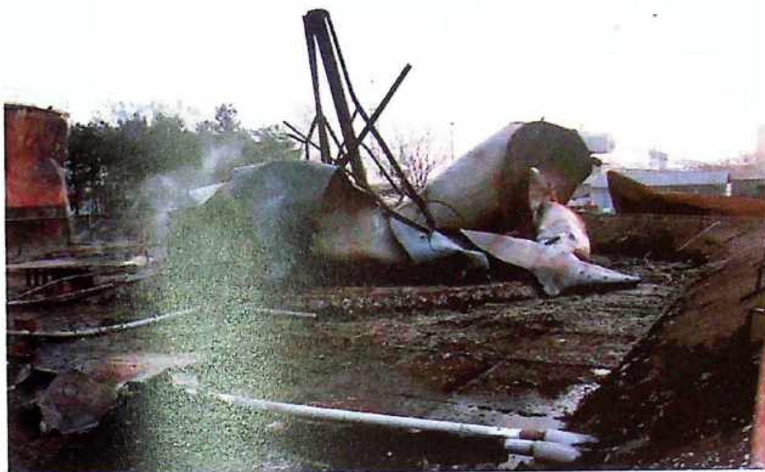
Photo 10 Burned oil storage tanks – "Beogradske elektrane", Novi Beograd
