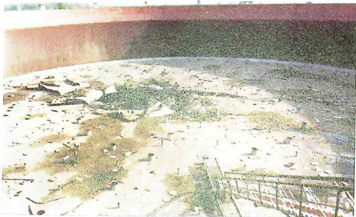
Photo 23 Damaged oil storage tank P-29
