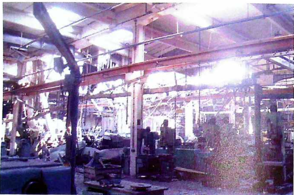
Photo 46 Damaged machinery in the Fittings and Fixtures Factory production plant
