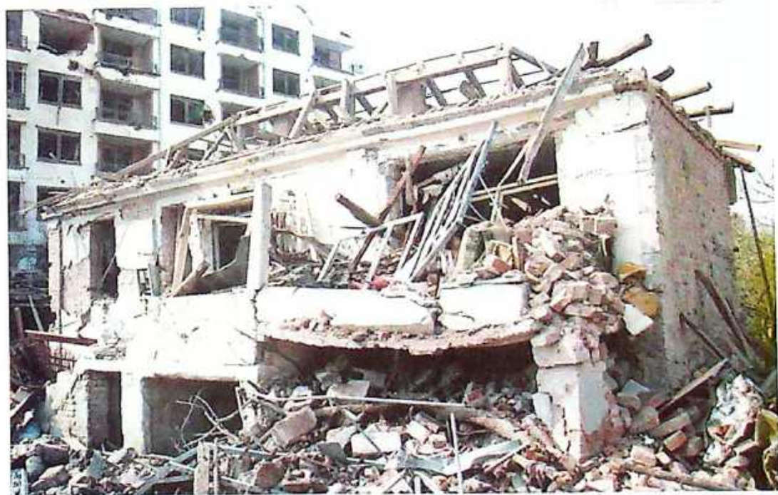
Photo 20 Demolished house on Dušan Trivunac St. in Aleksinac
