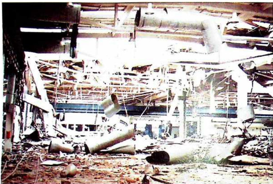
Photo 2 View of the damaged plant roof
