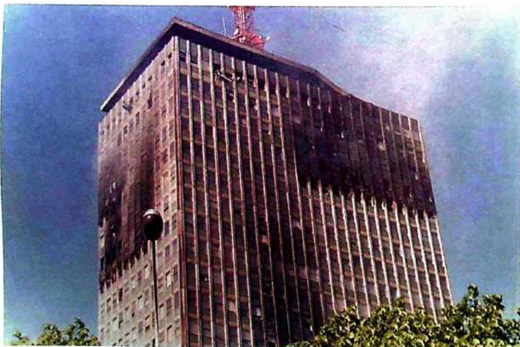
Photo 21 Upper floors of "Ušće" business center destroyed by fire
