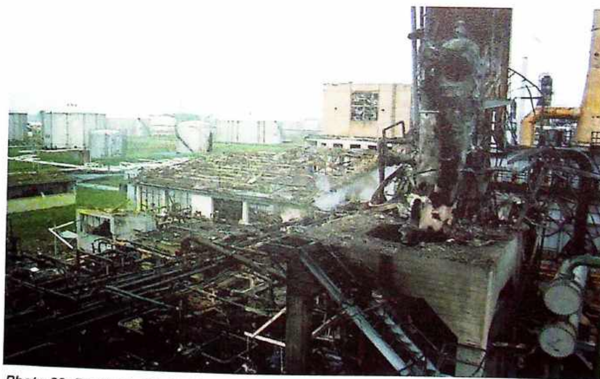
Photo 28 Bombed Oil Refinery in Novi Sad on 18 April 1999 - installation of atmospheric distillery AT-500 plant
