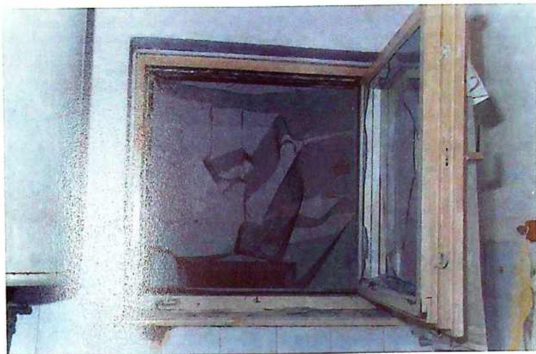
Photo 65 Damaged bathroom window
