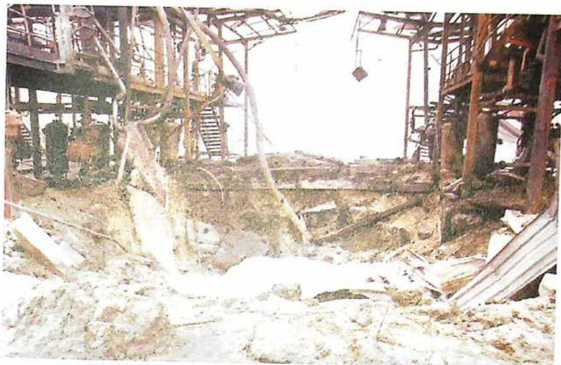
Photo 17 Demolished pouring station of NIS "Jugopetrol", Smederevo
