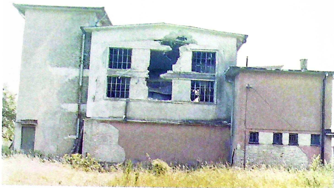
Photo 54 Bombed water supply centre "Jaroš" in Sombor, part of the public utility system "Vodokanal", May 30, 1999
