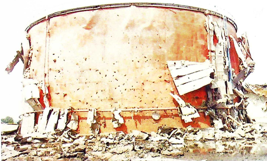
Photo 28 Damaged oil storage tank R-26 with torn off external insulation, NIS "Jugopetrol" – Instalacije, Smederevo, June 1, 1999
