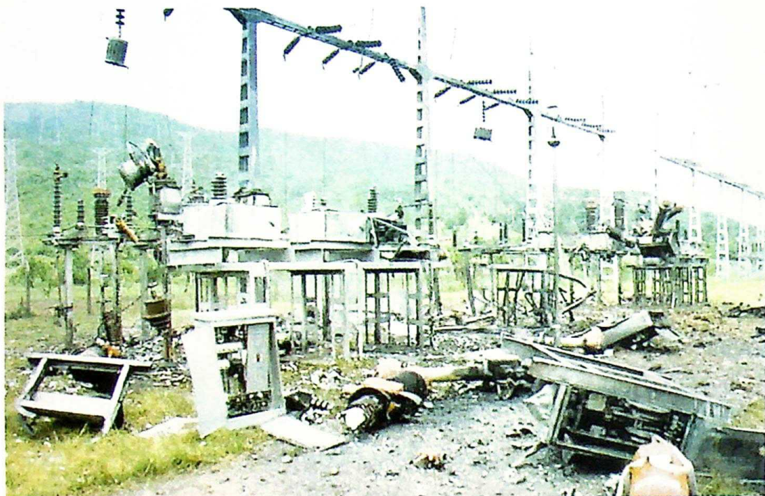
Photo 46 View of the damaged 110 kV electric installation of the public enterprise "Elektroistok" – Niš 2, in Niš, Bulevar Veljka Vlahovića St., May 23, 1999
