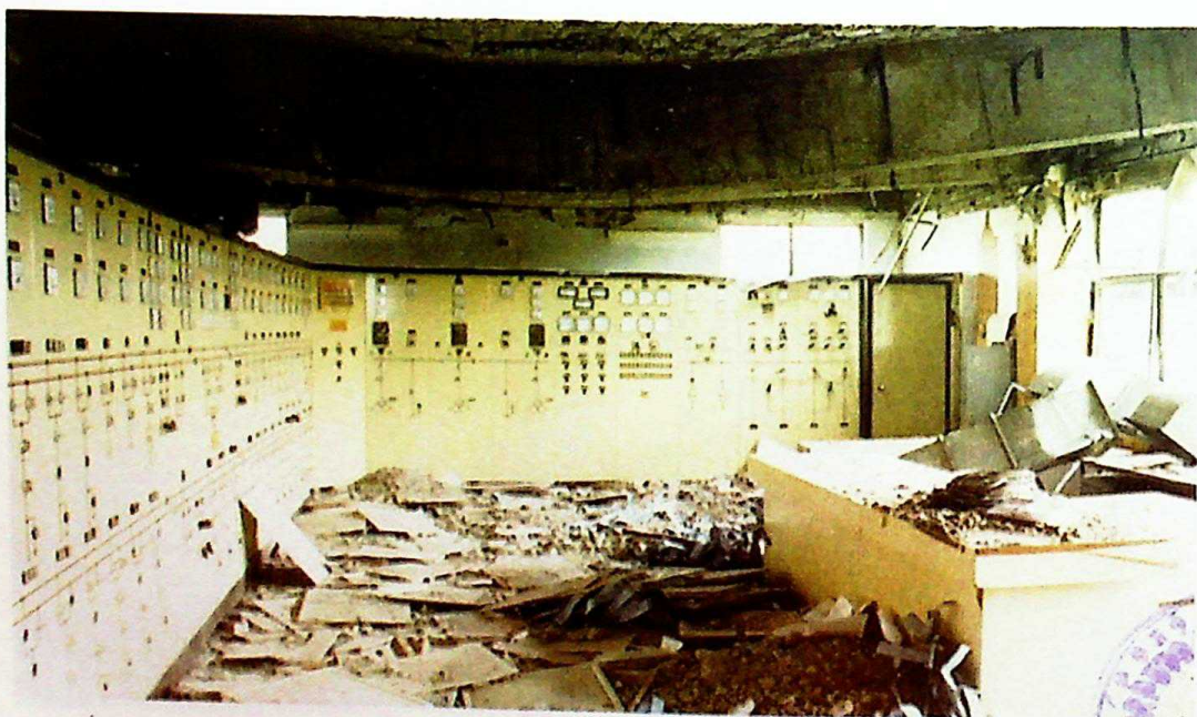
Photo 21 View of the damaged control room of No. 3 transformer station of RTB Bor, May 15, 1999
