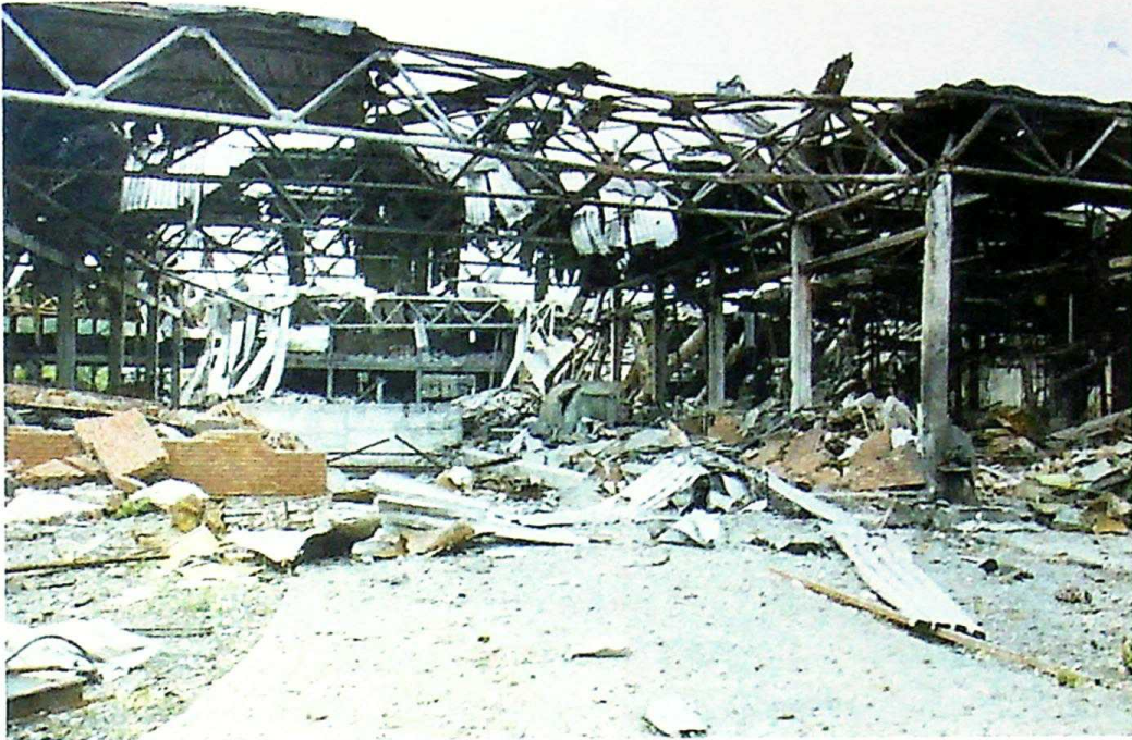
Photo 22 Demolished workshop of "Batteries" unit of DD "Krušik" Valjevo, May 18, 1999
