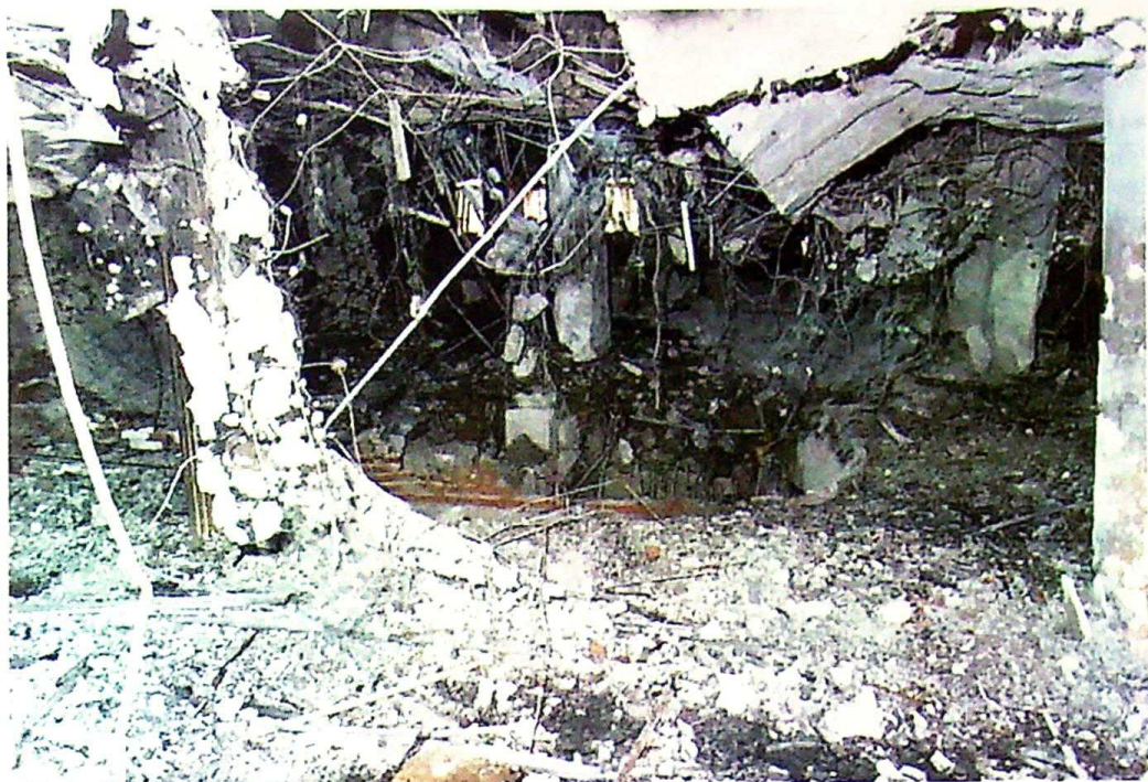
Photo 3 Close-up of one of the craters on the hotel ground floor
