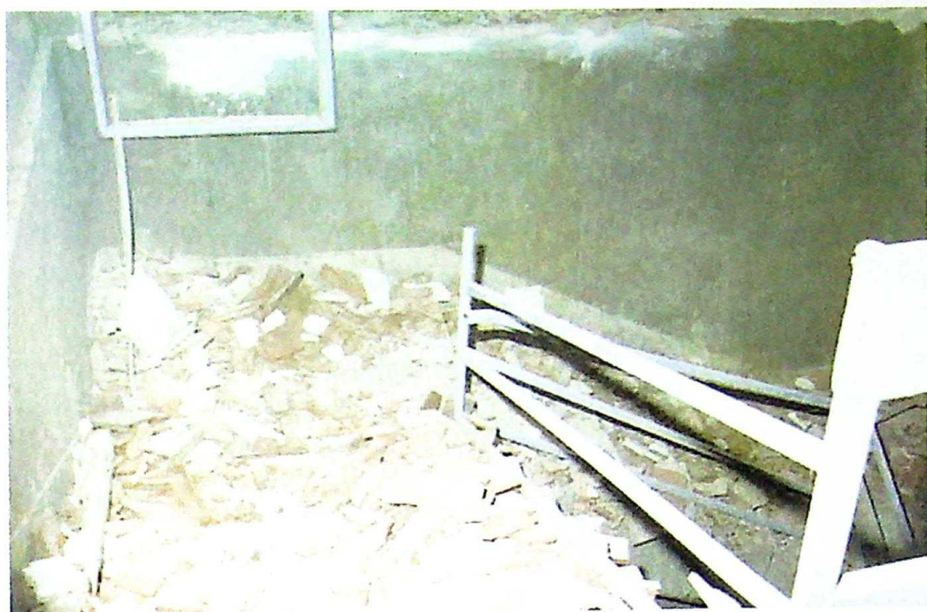
Photo 34 Ruined cellar of the "Mladost" company cafeteria where the killed female workers sought shelter on May 19, 1999
