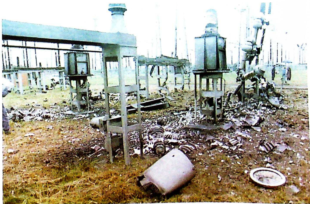
Photo 45 One of the damaged high-voltage fields in Urovci, May 23, 1999
