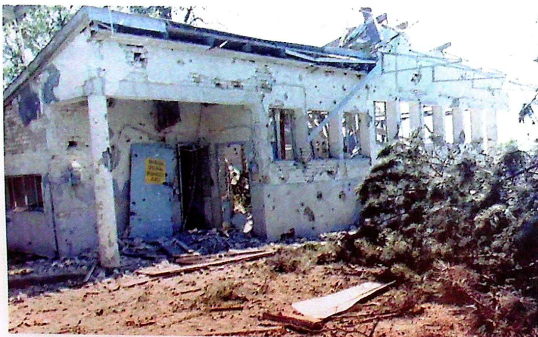
Photo 25 Destroyed old pump station in the storage area of NIS "Naftagas promet" in Sombor, May 21, 1999
