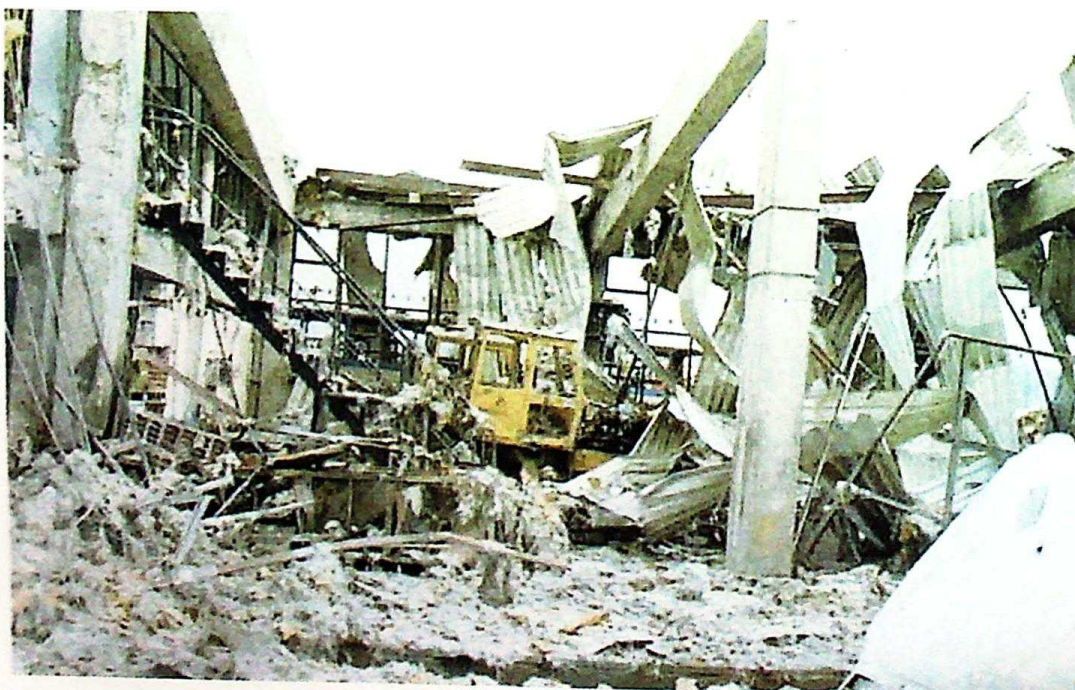
Photo 25 Close-up of the damaged "Machinery" unit of GP "Binačka Morava", Gnjilane, May 19, 1999
