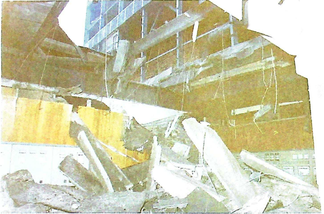
Photo 43 Point of the missile impact on the electric control centre of "Veliki Crljeni" power plant
