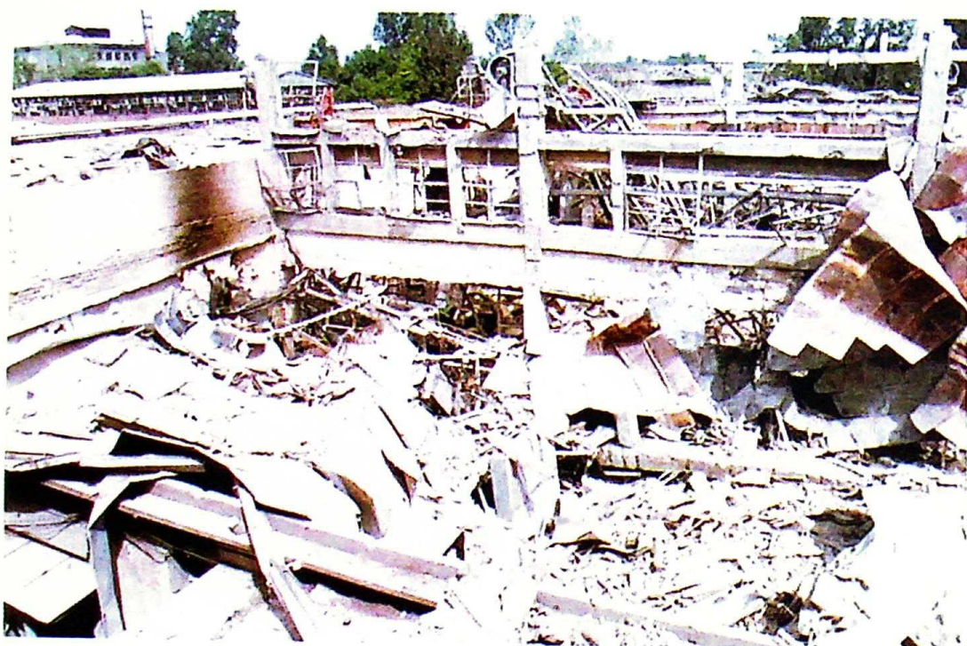
Photo 17 Demolished processing equipment workshop of HK "Prva Iskra" Barič
