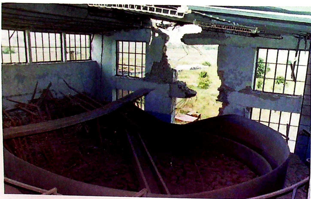
Photo 55 Close-up of the destroyed tank in the water-pumping station of the water supply centre "Jaroš" in Sombor, May 30, 1999
