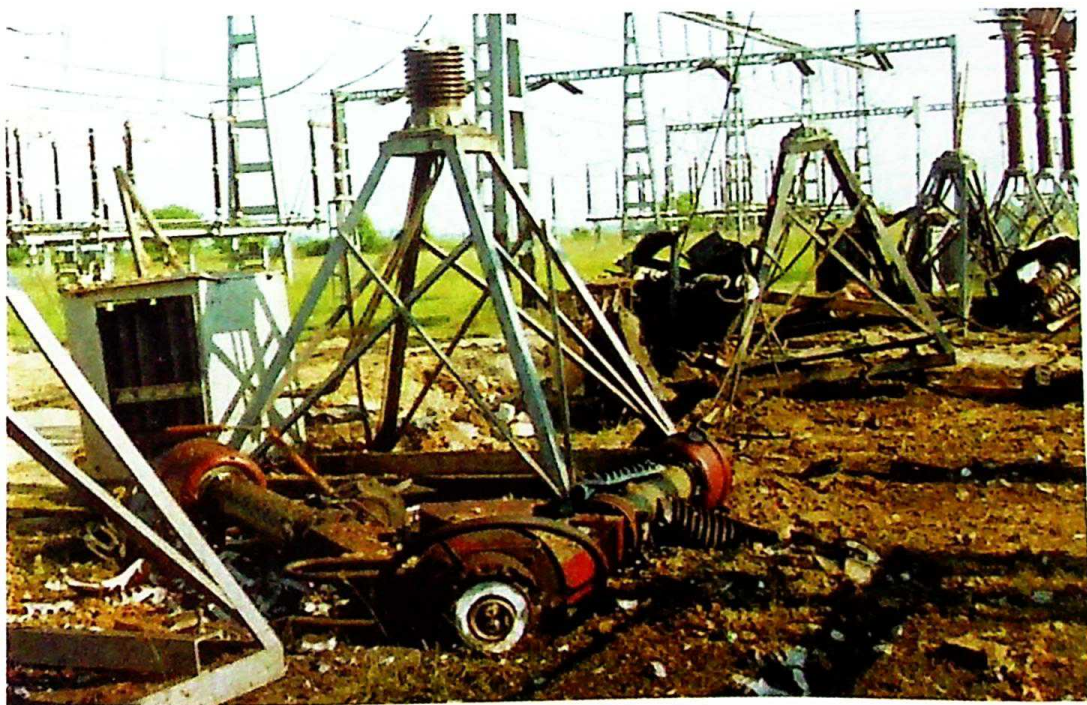
Photo 49 View of the wrecked 380 kV installation of "Novi Sad 3" transformer station, May 24, 1999
