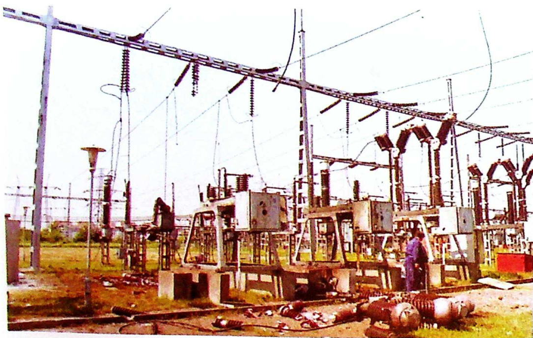
Photo 51 Damaged electric installation of the 220 kV "Beograd 5" transformer station on Bežanijska Kosa
