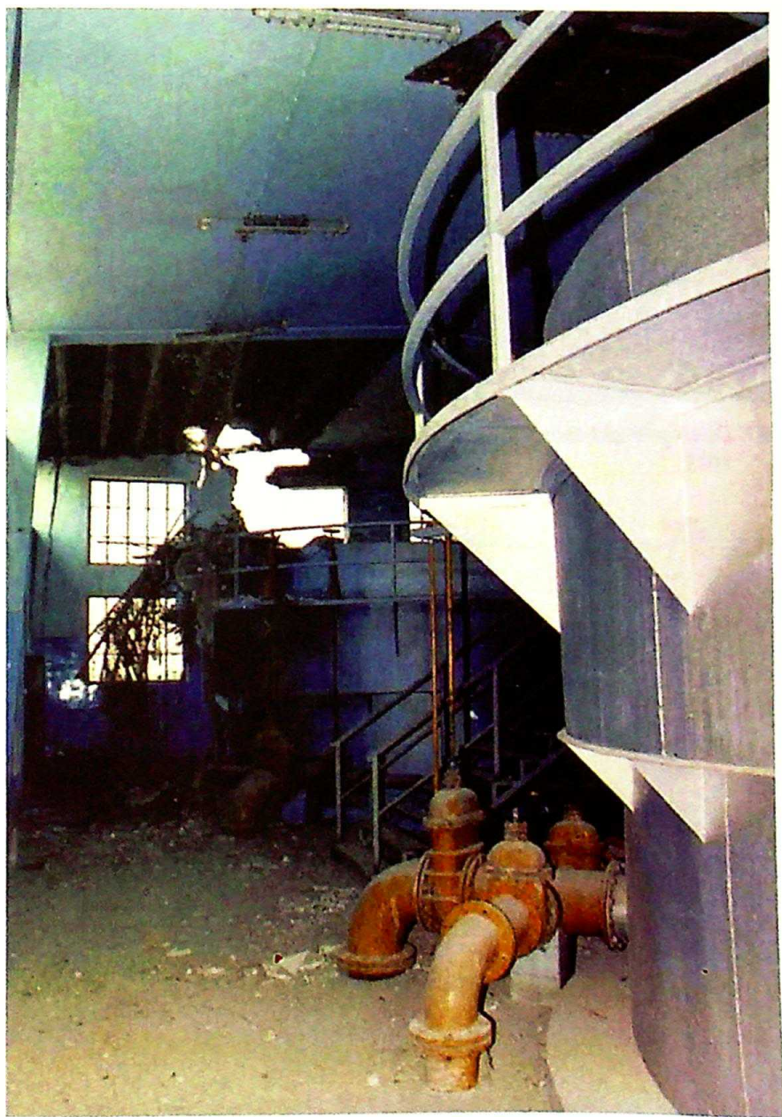
Photo 56 Interior of the water-pumping station "Jaroš" in Sombor, May 30, 1999
