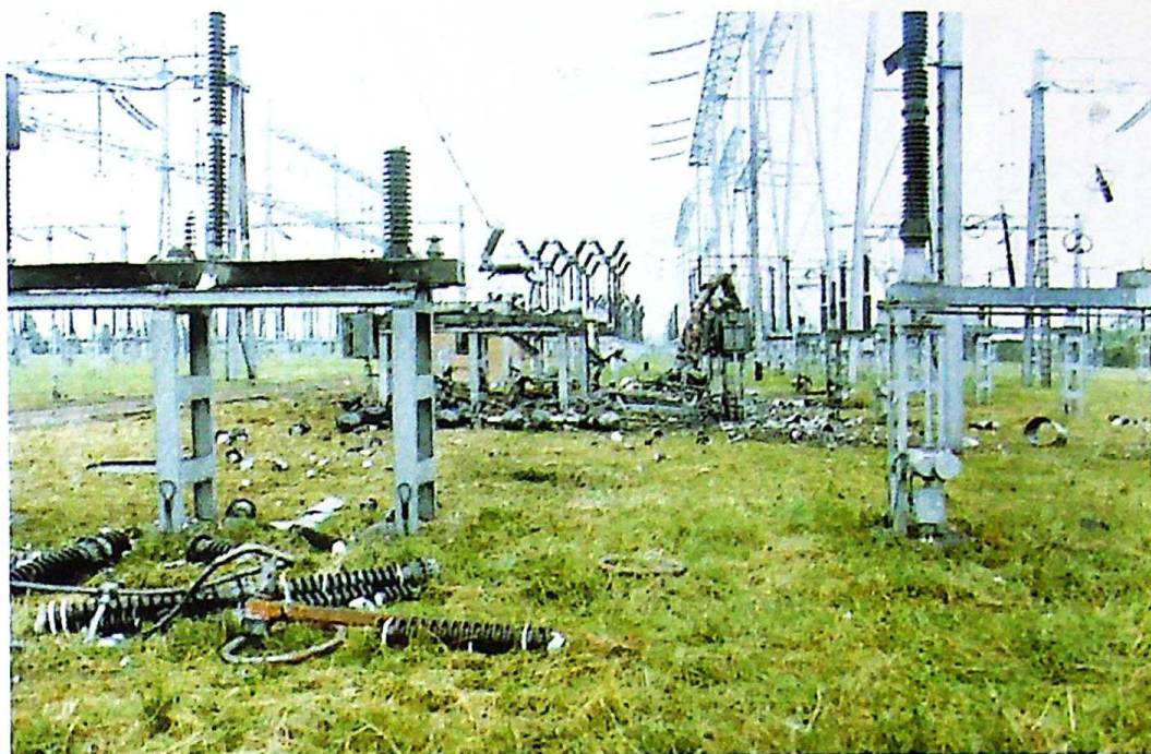
Photo 44 Damaged high-voltage distributor installation of thermal electric power plant A in Urovci–Obrenovac, May 23, 1999
