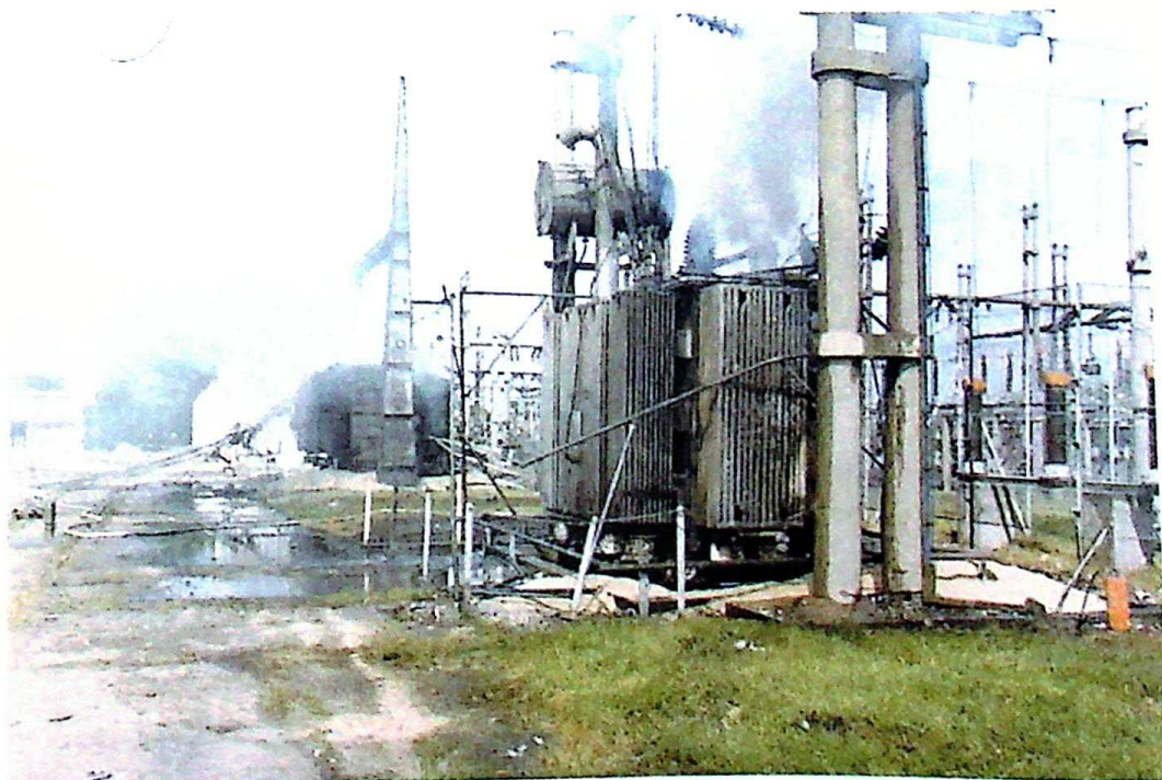
Photo 42 Damaged block transformers of "Veliki Crljeni" power plant
