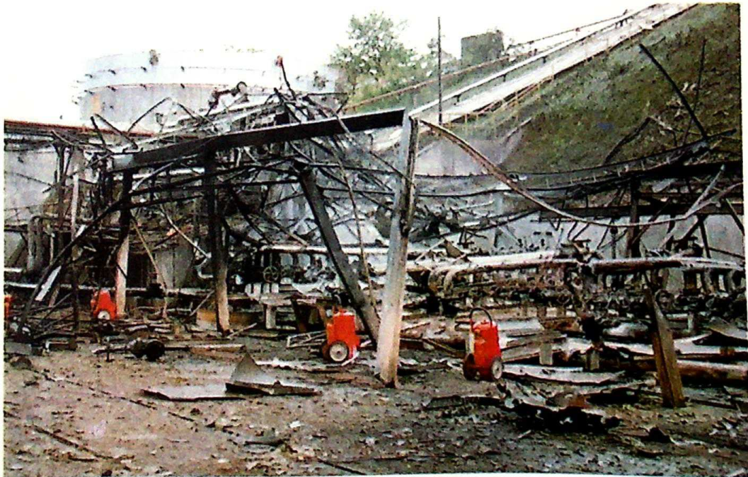
Photo 8 Demolished pump station No. 1 of "Jugopetrol" – Beograd, Prahovo-Bor installation, May 7, 1999 (1st attack)
