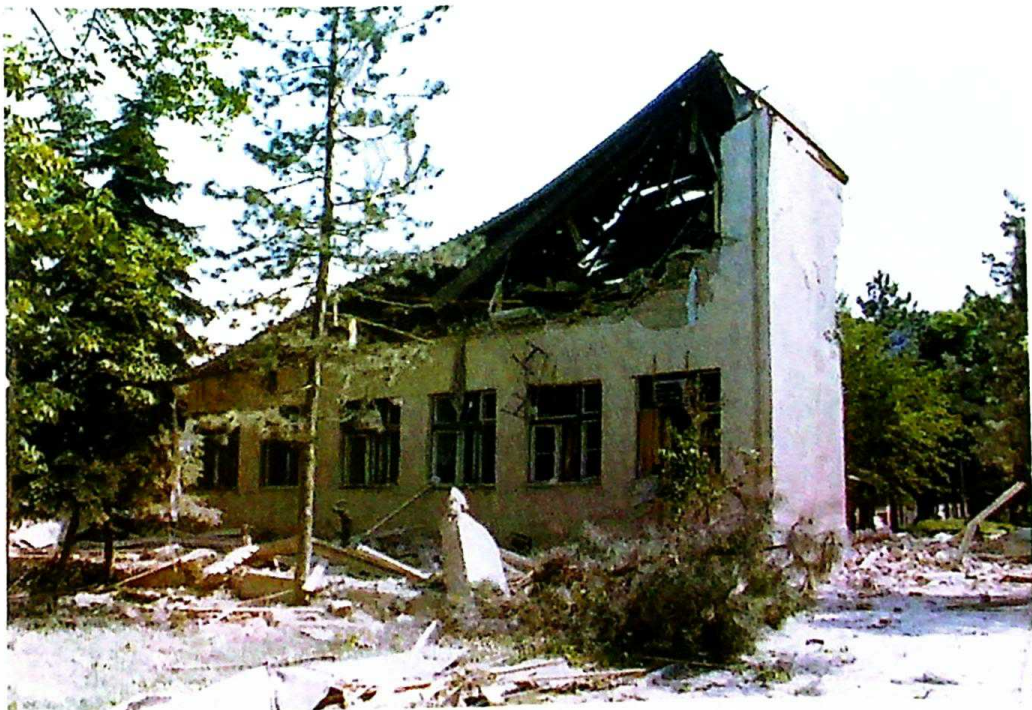
Photo 16 Destroyed administration building of HK "Prva Iskra" Barič, May 10, 1999
