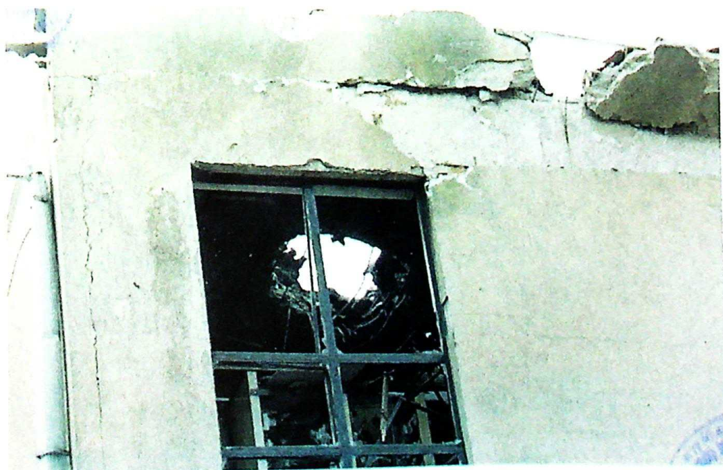
Photo 19 Hole in the ceiling of No. 3 transformer station building of RTB Bor where the missile came through
