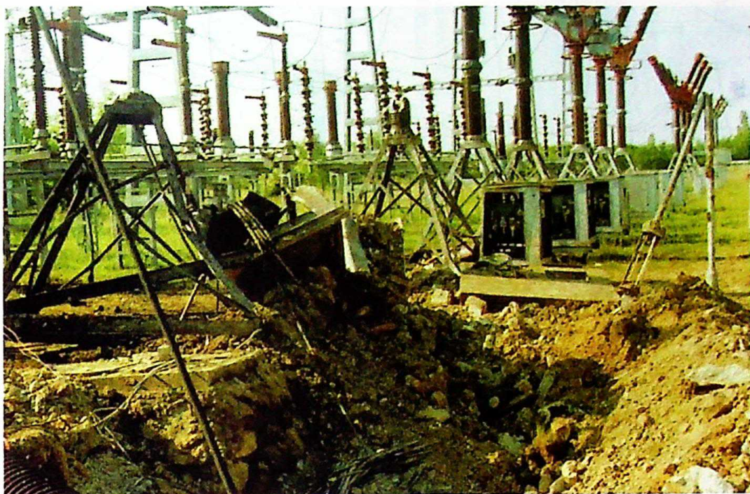
Photo 48 Point of the missile impact on "Novi Sad 3" transformer station (Rimski šančevi), May 24, 1999
