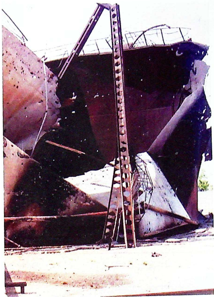
Photo 22 Destroyed oil storage tank No. 3 in the central storage area of NIS "Naftagas promet" in Sombor, F. Kljajić Street, May 20, 1999
