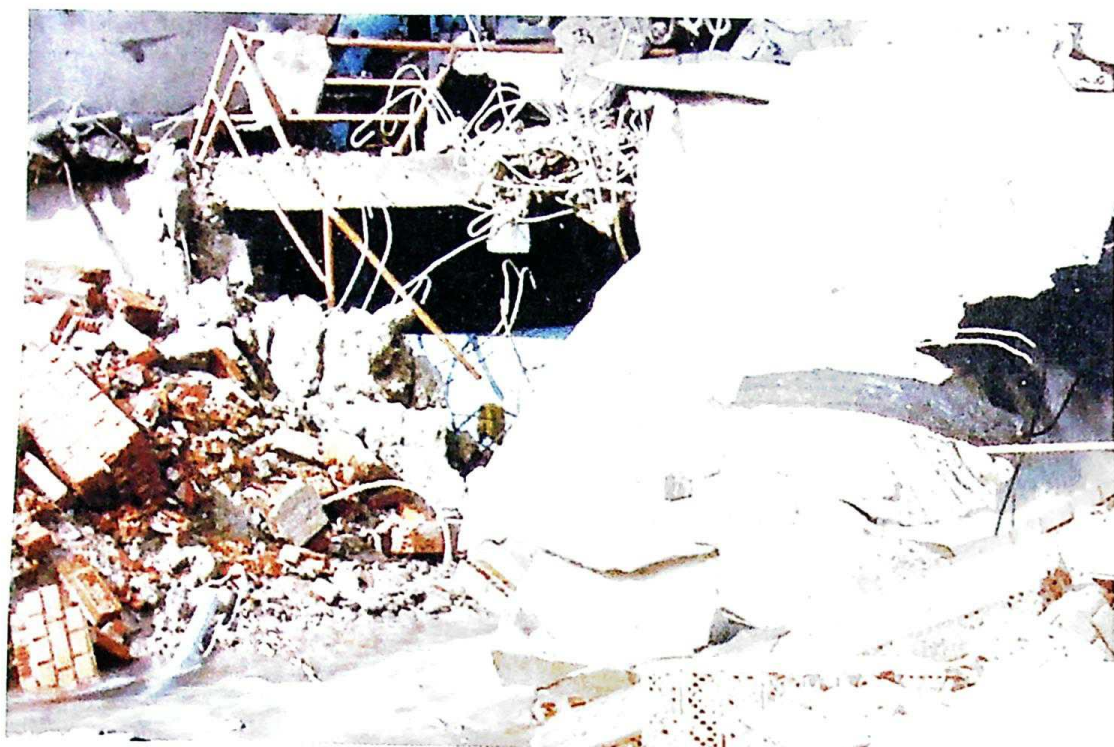
Photo 2 Close-up of the "Badovac" water-pumping station
