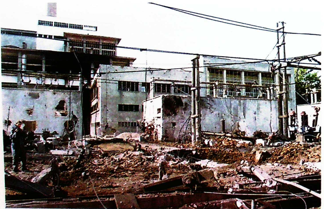
Photo 40 Destroyed energy field of the generator No. 1 and the administration building of "Veliki Crljeni" power plant, Lazarevac, May 22, 1999
