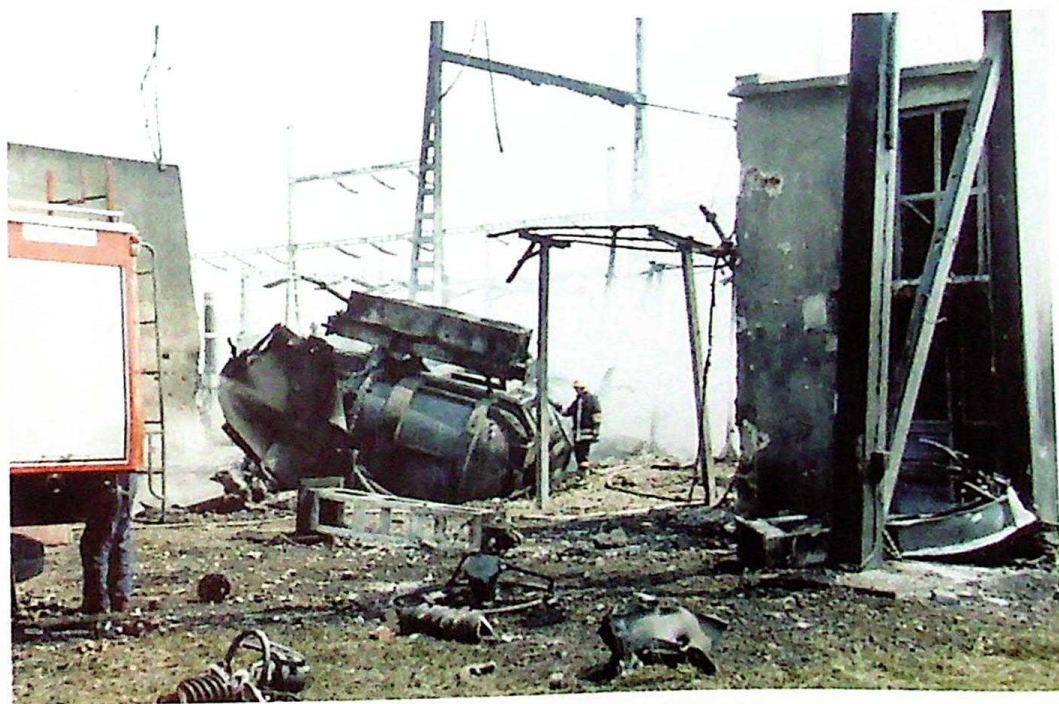
Photo 60 View of one of the destroyed transformers of "Transformer Station 3", May 31, 1999
