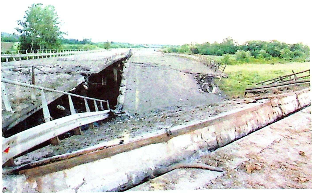
Photo 76 Close-up of the torn down bridge over the river Jasenica
