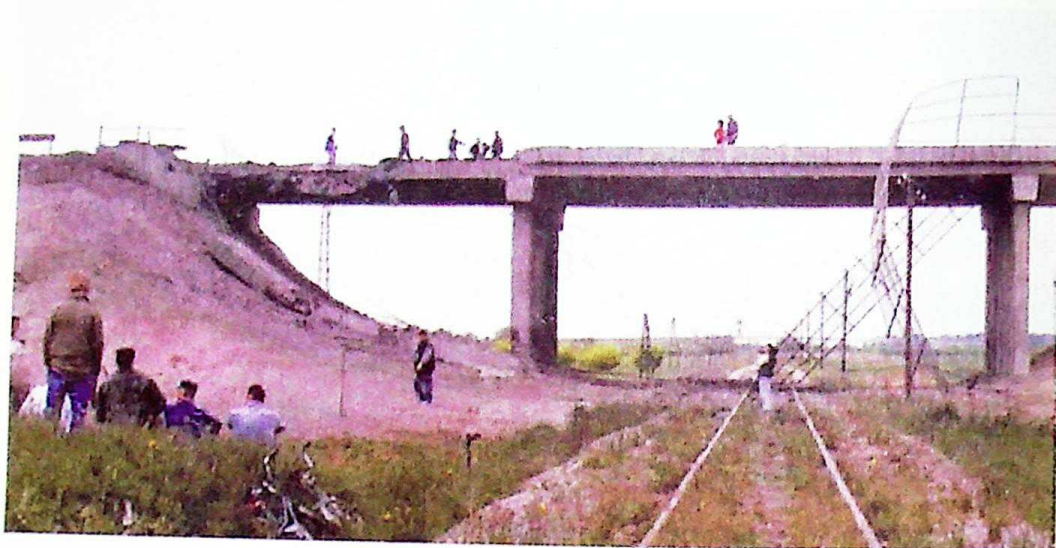
Photo 55 Damaged Horgoš flyover on the E-75 motorway and the damaged railway Subotica–Horgoš–Szeged, May 11, 1999
