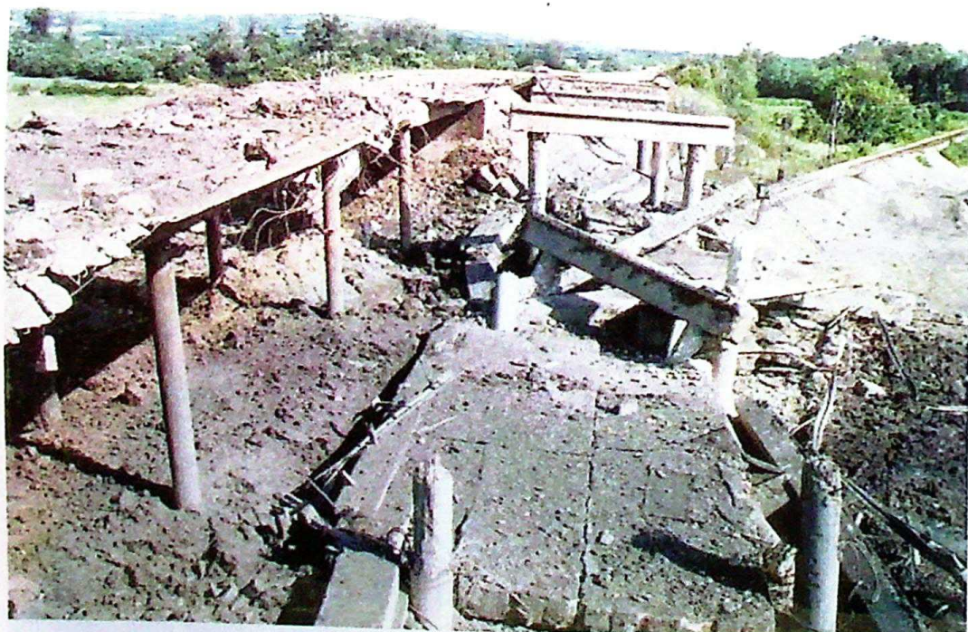
Photo 111 Close-up of the demolished flyover near V. Plana, June 2, 1999
