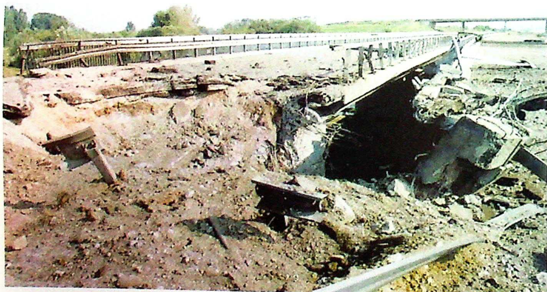
Photo 90 Close-up of the damaged bridge over the river Nišava, May 28, 1999
