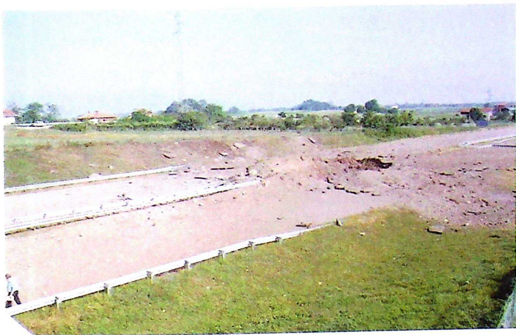
Photo 91 Damaged motorway Belgrade–Niš–Leskovac in the area of the village of Popovac–Niš, May 28, 1999 (view from the flyover from the direction of Niš)
