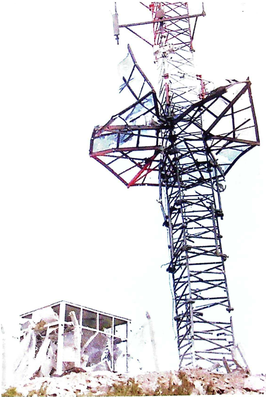
Photo 31 Damaged antenna pole and the demolished "Mobtel" container on "Gobelja", Mt. Kopaonik, June 3, 1999
