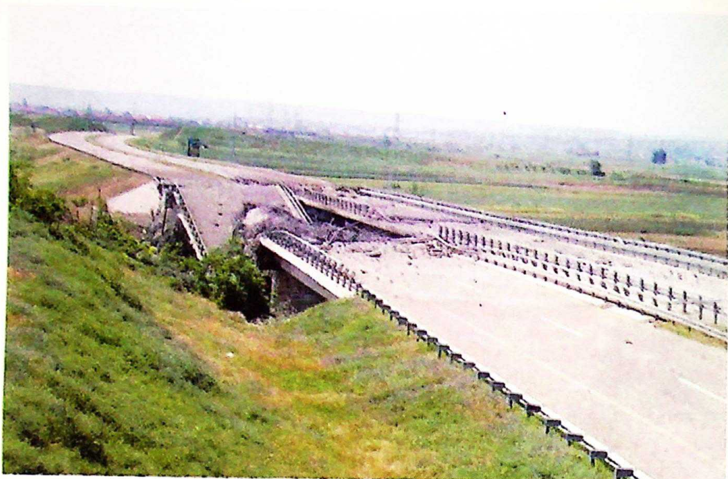
Photo 93 Torn down section of the bridge over the river Nišava on the Belgrade–Niš–Leskovac motorway in the village of Popovac–Niš, May 30, 1999 (2nd
