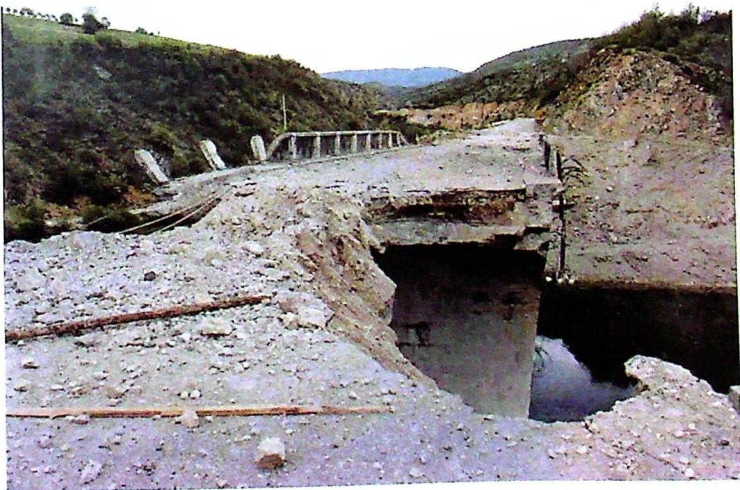
Photo 58 Close-up of the damaged bridge in Kokin brod, May 11, 1999
