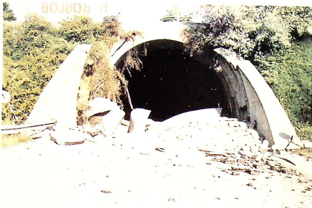
Photo 106 Bombed tunnel leading to the "Sloboda" bridge from Sremska Kamenica to Novi Sad, May 30, 1999
