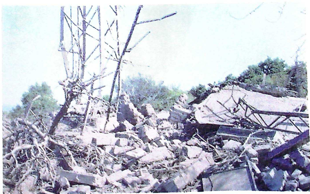
Photo 24 Completely destroyed building and damaged antenna pole of the repeater on Kozarica hill–Dimitrovgrad, May 30, 1999
