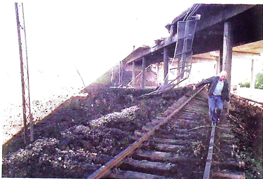
Photo 49 The damaged Belgrade–Velika Plana railway under the motorway flyover
