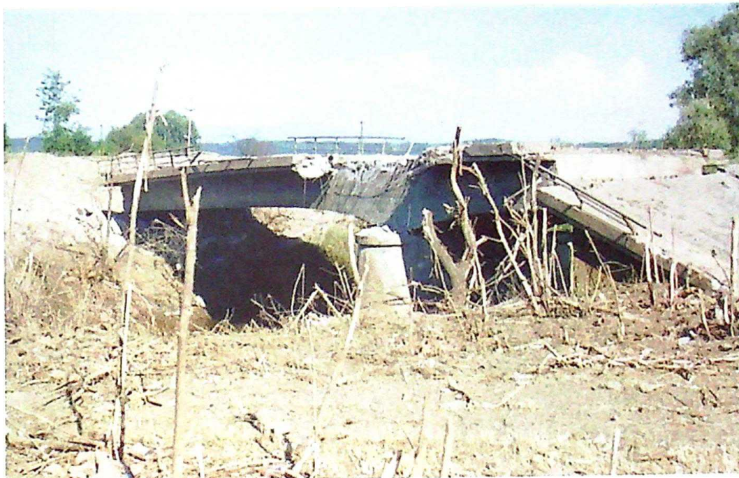
Photo 83 Destroyed Čenovački bridge on the river Jablanica in Čenovac, municipality of Lebane – Leskovac, bombed on 29 May 1999 and 30 May 1999
