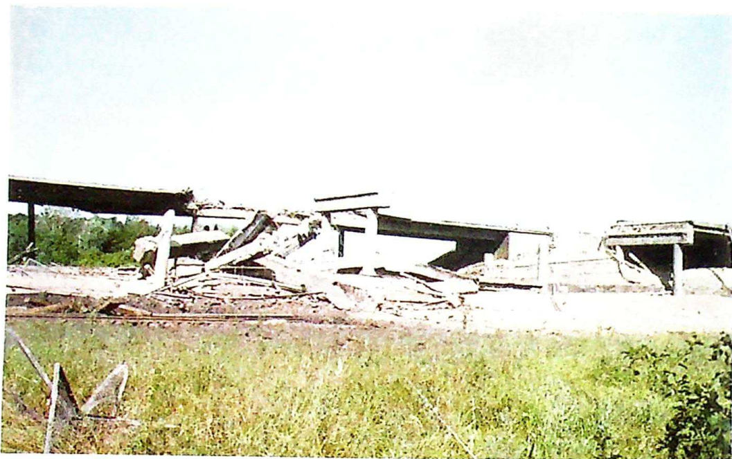
Photo 110 Demolished flyover on the Belgrade–Niš motorway, the area of the village Orašje, which collapsed on the Belgrade–V. Plana railway tracks on June 2, 1999, V. Plana (3rd attack)
