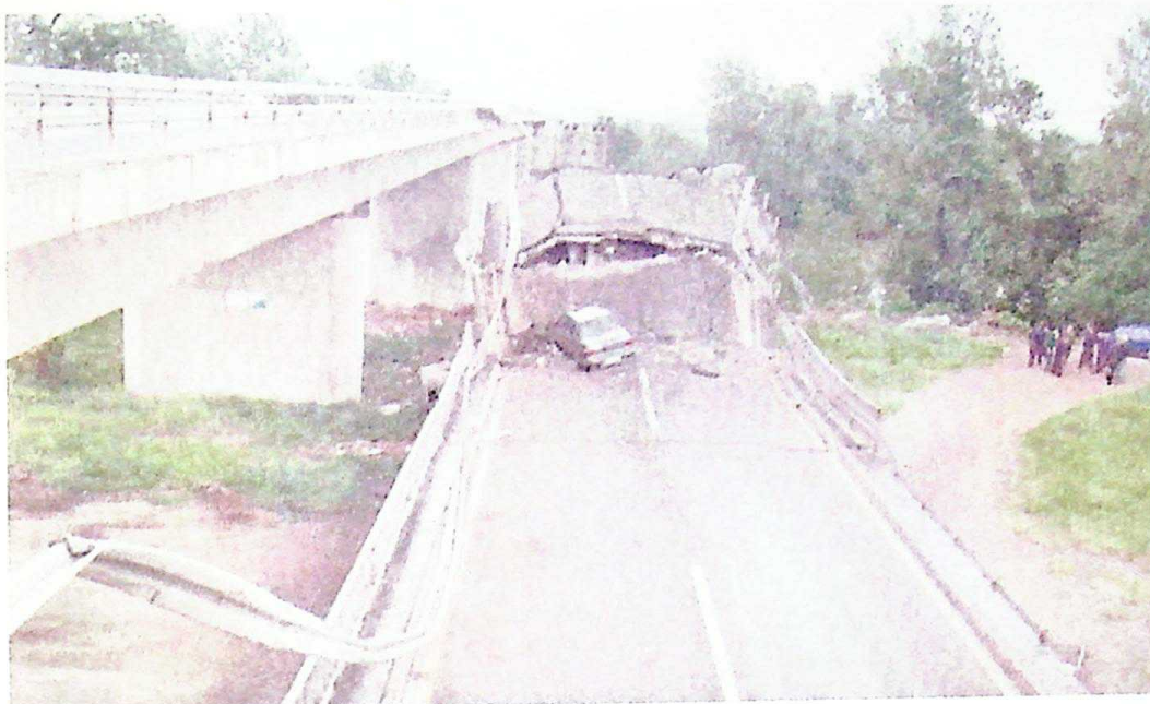
Photo 43 Destroyed right-hand side lane of the bridge over the river Nišava, near Mijatovac village – Čuprija, on the Belgrade–Niš motorway, May 8, 1999 (viewed from the direction of Belgrade)
