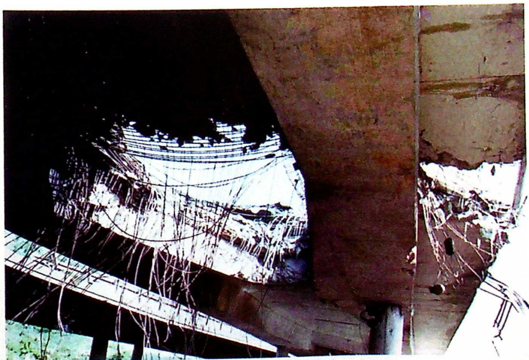
Photo 113 Craters on the bridge over the river Jasenica in V. Plana, June 2, 1999
