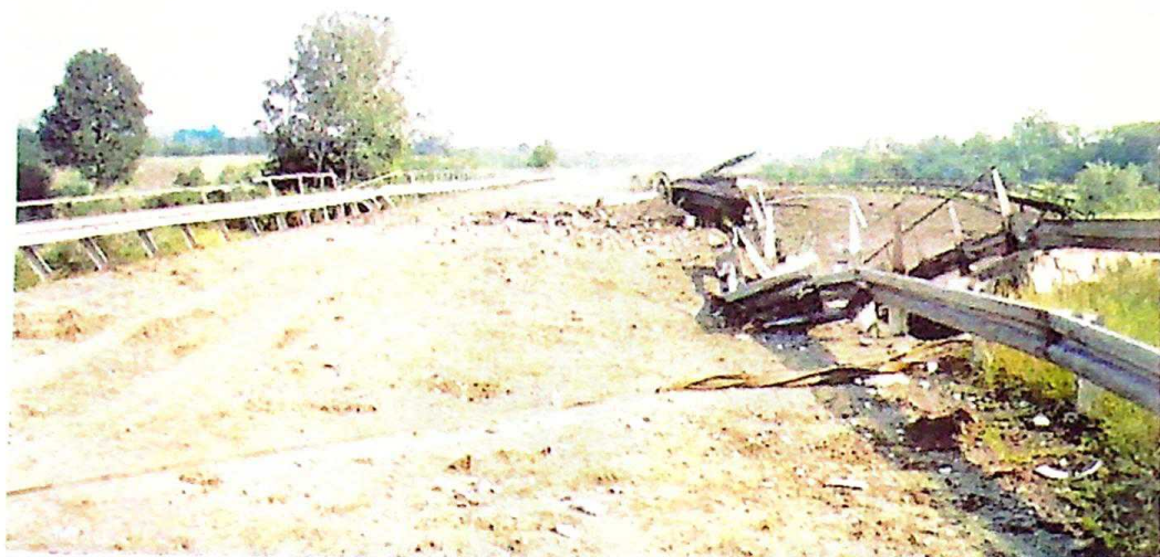
Photo 77 Bombed left side of the bridge over the river Jasenica on the Belgrade-Niš motorway (driving lane from the direction of Niš) in Velika Plana, May 26, 1999 (4th attack)
