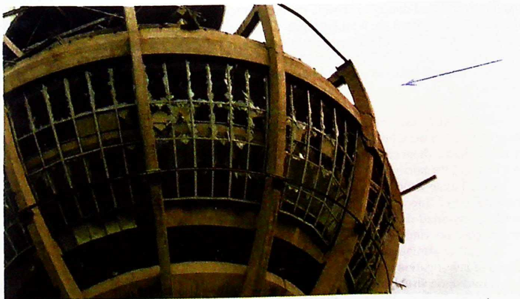
Photo 2 View of the dome of the bombed radio and TV transmitter tower of RTS on Iriški Venac, April 28, 1999 (2nd attack)
