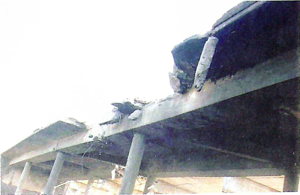
Photo 47 The damaged flyover on the Belgrade–Niš motorway, near Velika Plana, May 10, 1999
