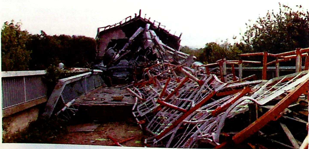
Photo 4 View of the destroyed 120 m high antenna pole on Mt. Avala
