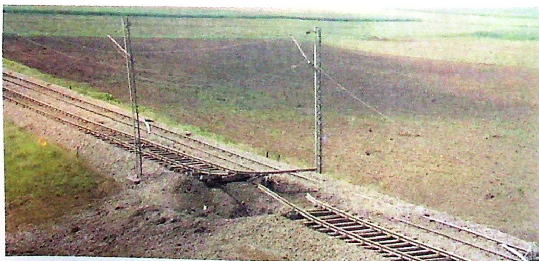
Photo 67 Broken railway tracks on the Belgrade–Skoplje railway line in the vicinity of the demolished flyover near Trupalske forests – Niš, May 14, 1999
