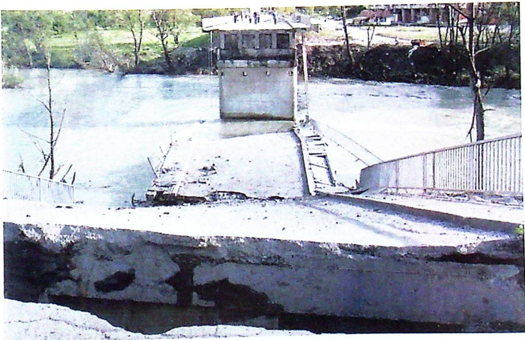
Photo 54 Demolished bridge over the river Lim in Prijepolje on the main road Prijepolje – Užice, May 11, 1999 (Second attack)
