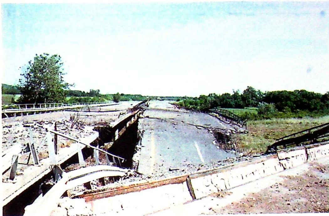
Photo 112 Bombed bridge over the river Jasenica on the Belgrade–Niš motorway, near V. Plana, June 2, 1999 (3rd attack)
