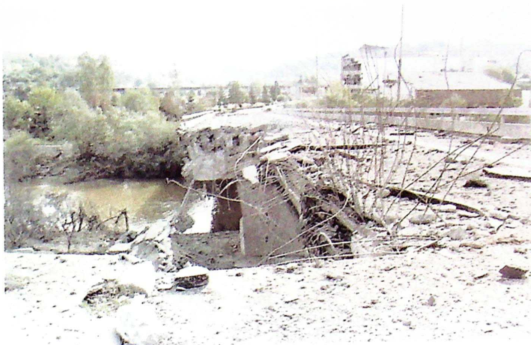
Photo 68 Bombed bridge over the river Južna Morava in Vladičin Han downtown, viewed in the direction of Surdulica, May 18, 1999
