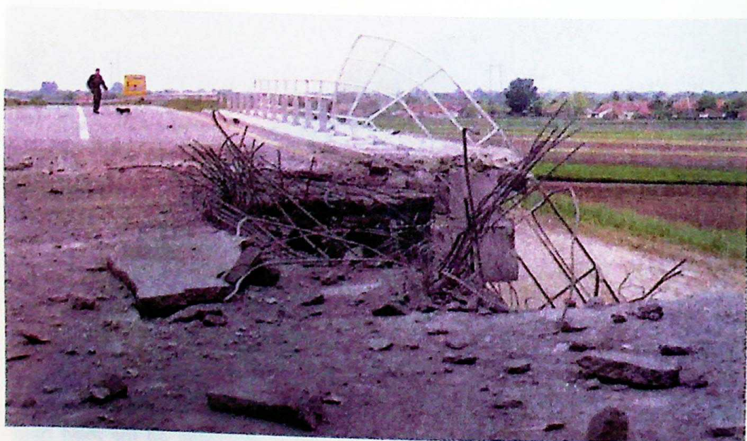
Photo 56 Close-up of the damage on the Horgoš flyover, May 11, 1999
