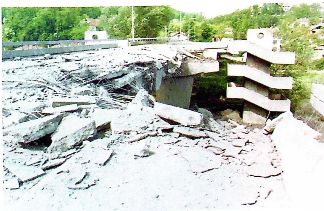
Photo 69 Damaged mid-section of the bridge over the river Južna Morava in Vladičin Han
