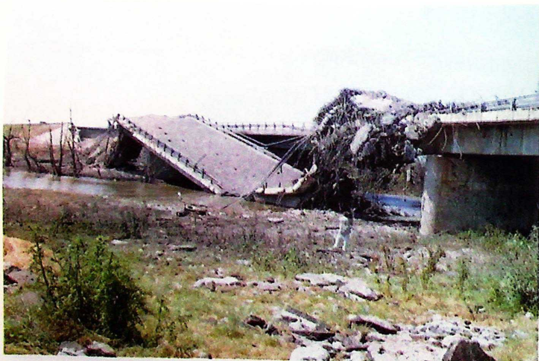
Photo 94 Close-up of the destroyed section of the bridge over the river Nišava
