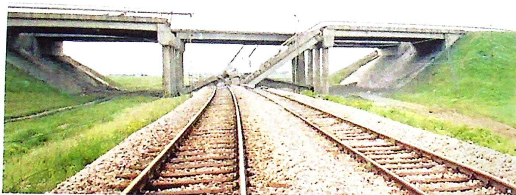
Photo 66 The flyover on the Belgrade–Skoplje motorway, near Trupalske forests, which collapsed on the Belgrade–Skoplje railway tracks in the vicinity of Niš, May 14, 1999
