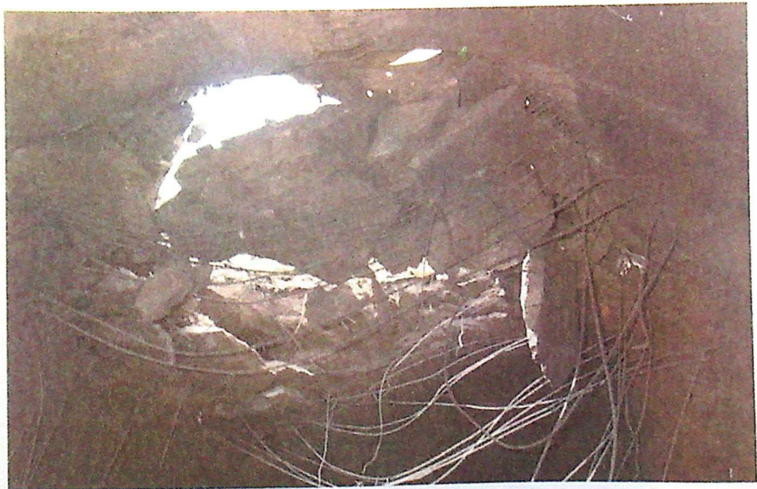
Photo 109 One of the craters caused by a missile impact, viewed from inside the tunnel, May 31, 1999
