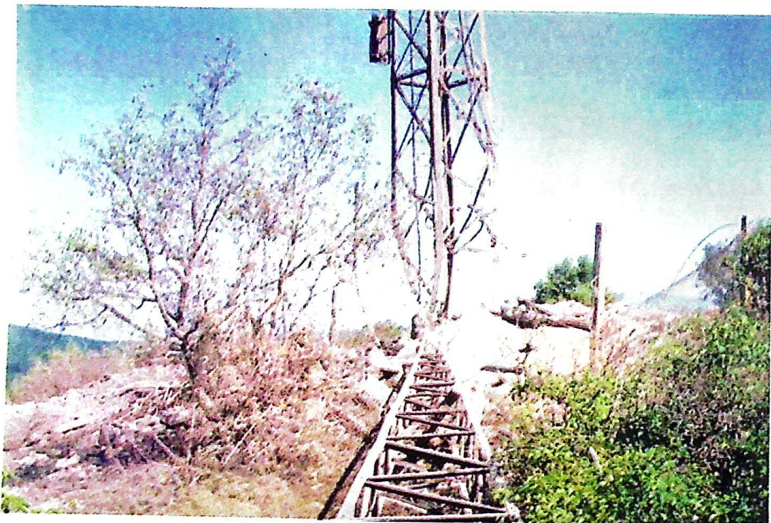
Photo 25 Damaged antenna pole of the radio and TV repeater on Kozarica hill—Dimitrovgrad, May 30, 1999
