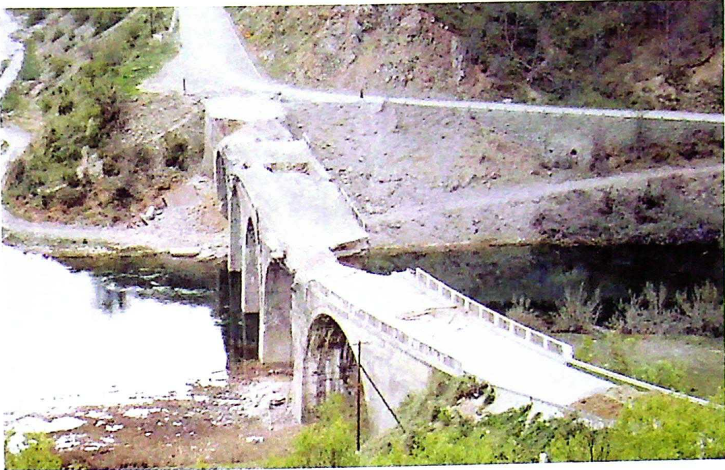
Photo 57 Bombed bridge over the river Uvac in Kokin brod, on the Nova Varoš–Užice road, May 11, 1999 (second attack)
