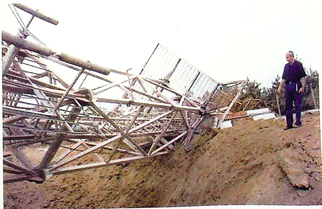
Photo 18 Close-up of the toppled antenna pole of the repeater on Mt. Cer, May 20, 1999.
