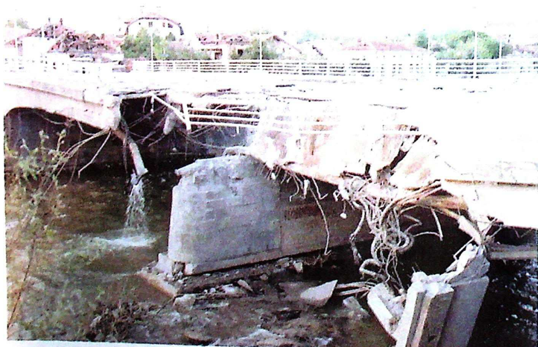
Photo 42 Close-up of the demolished bridge on the river Nišava
