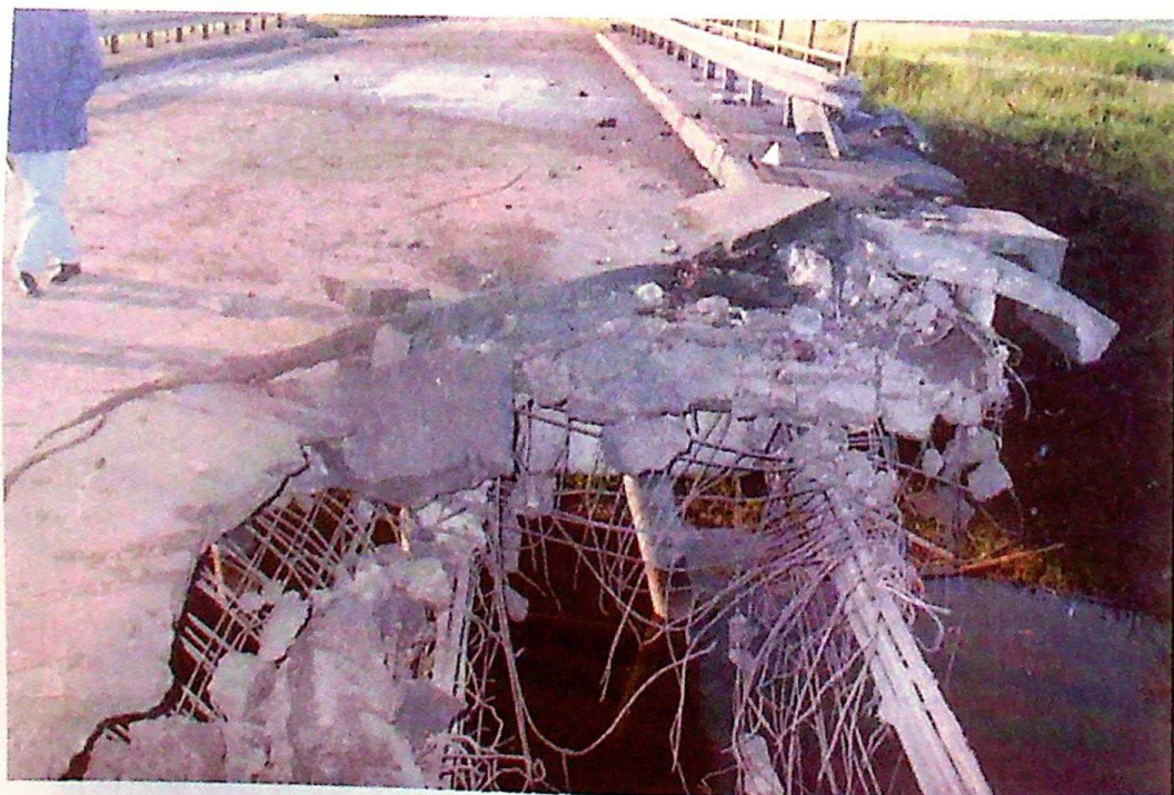
Photo 74 Close-up of the damaged bridge over the Stari Begej
