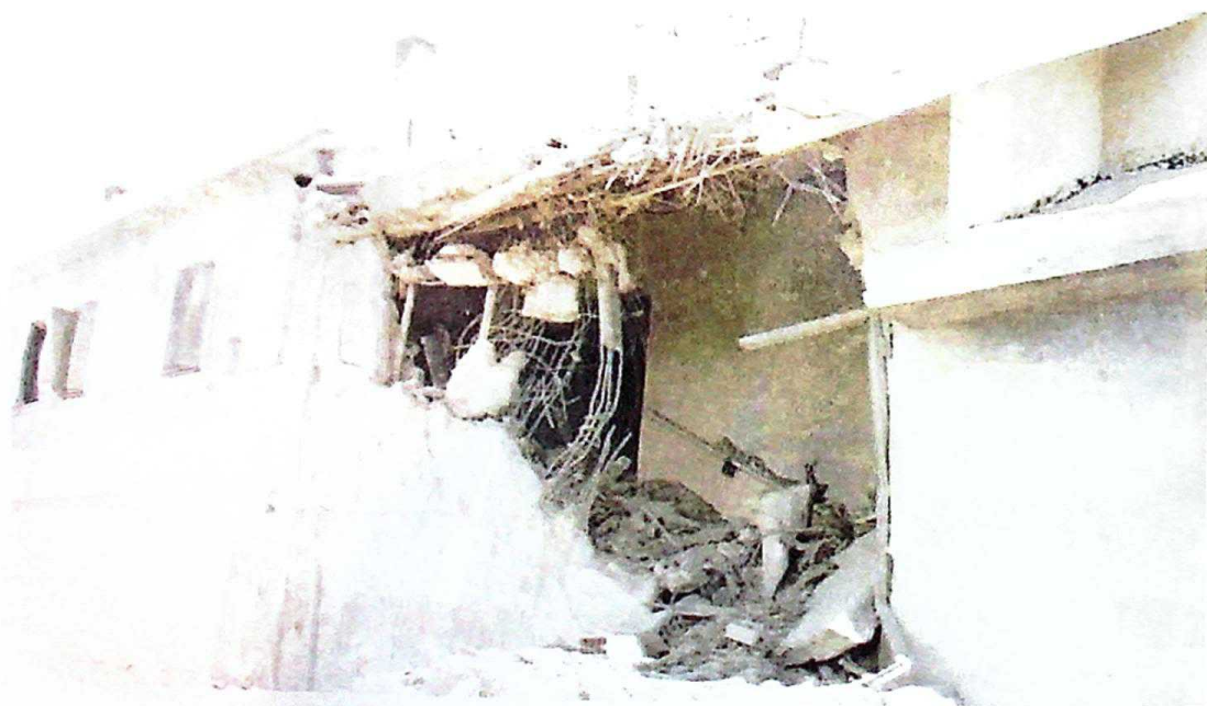
Photo 22 Point of the missile impact on the RTS repeater building on Mt. Besna Kobilica–Vranje, May 30, 1999
