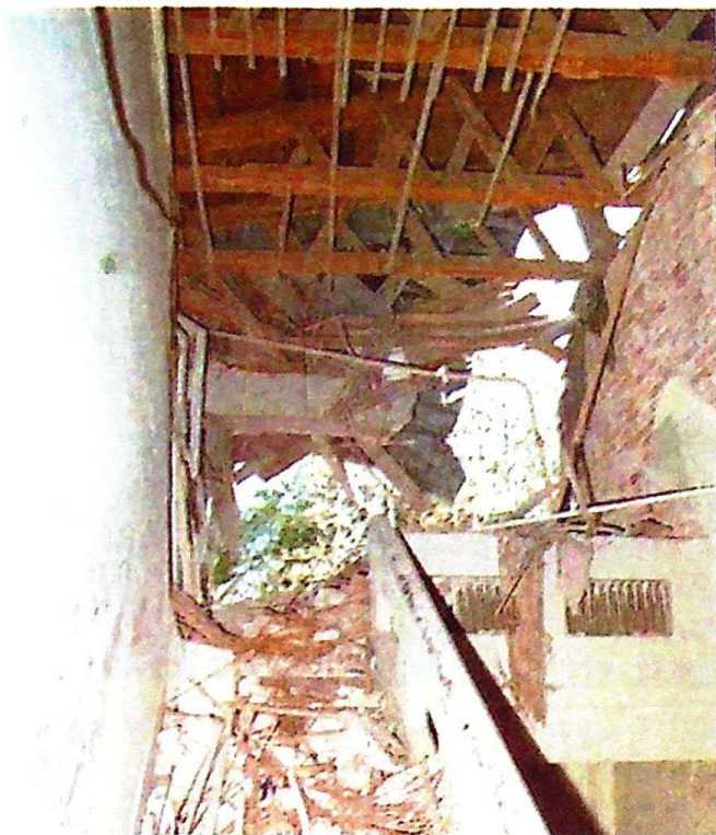
Photo 15 The stairway of the bombed "Sanatorium" building
