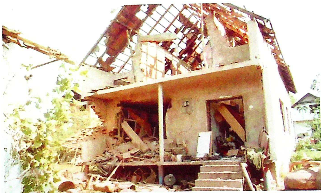
Photo 120 Destroyed houses at No. 10 Užička St., Aleksinac, property of Miroslav Rašić. On 28 May 1999, about 80 houses were destroyed or damaged in Aleksinac, almost all of them on Užička St. and Niška St.
