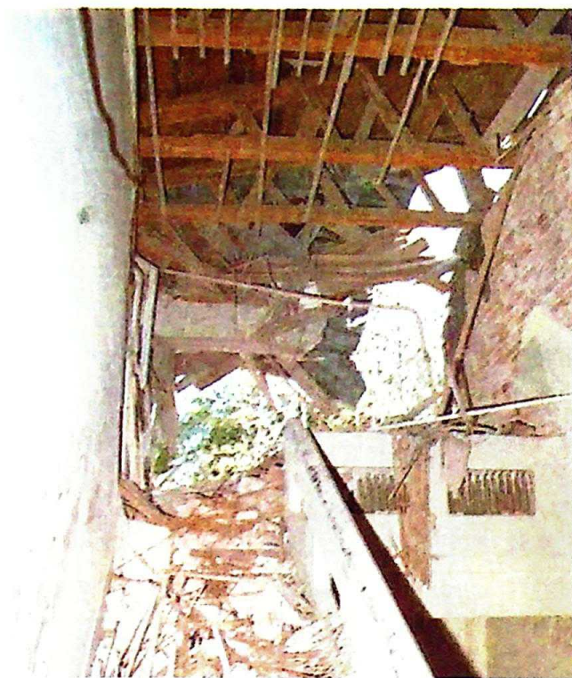
Photo 15 The stairway of the bombed "Sanatorium" building
